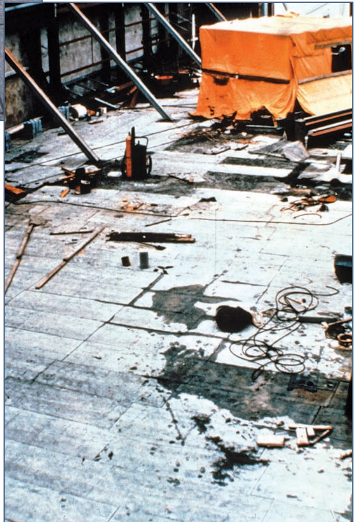
Photo 10 – Typical construction abuse after installation.
