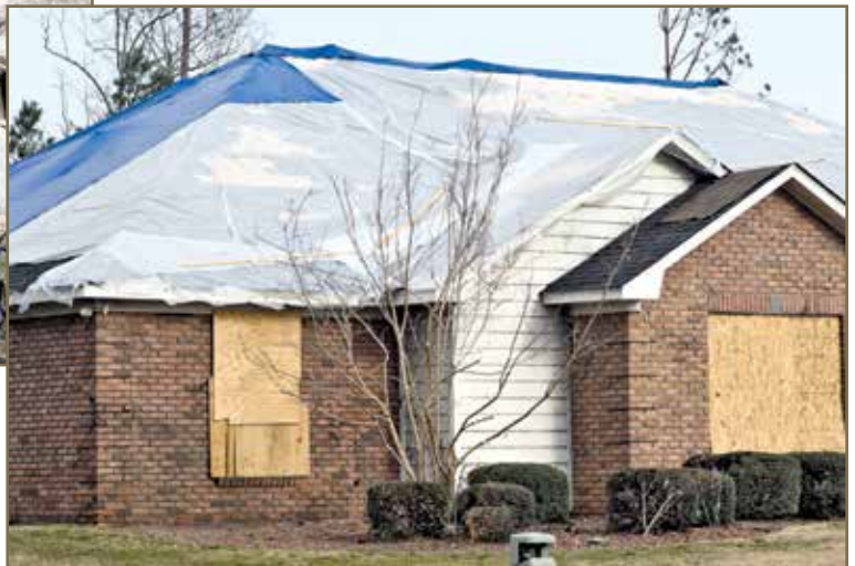
Photo 3 – House is still standing, but the roof has been torn off.
