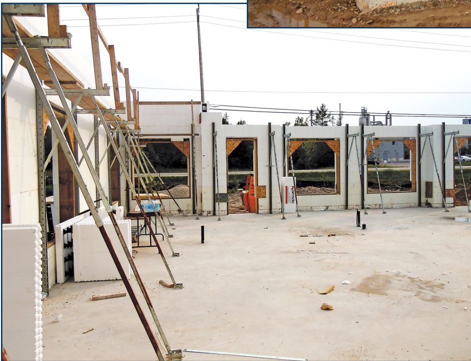
Figure 5 – Temporary braces are placed around the interior of the walls before pouring, in order to keep the walls plumb during concrete pouring.
