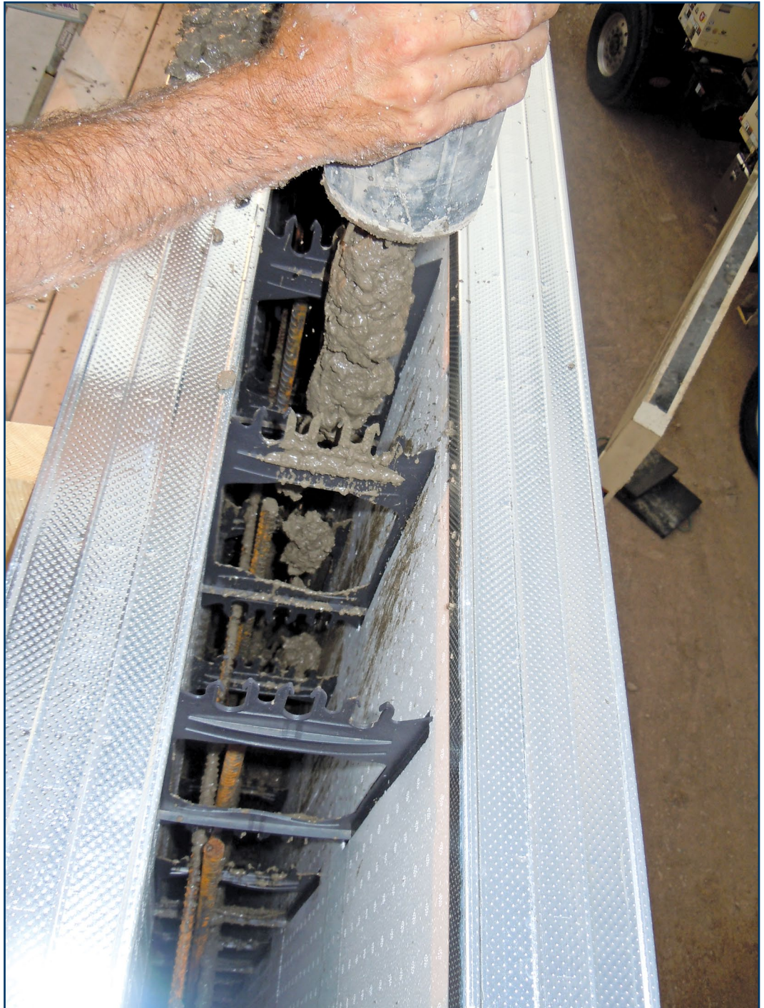
Figure 2 – Concrete is pumped into the ICFs, filling in around the reinforcement and webs, creating a solid concrete wall. (Image courtesy of Roylton Construction.)
