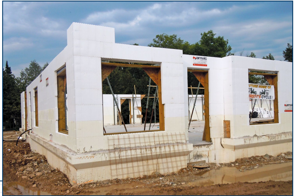
Figure 4 – The foundation of this project was formed with 2.5-in. ICF, and the above-grade walls with 3.25-EPICF blocks. The foundation is seen here partially exposed. It was later backfilled up to the brick ledge.
