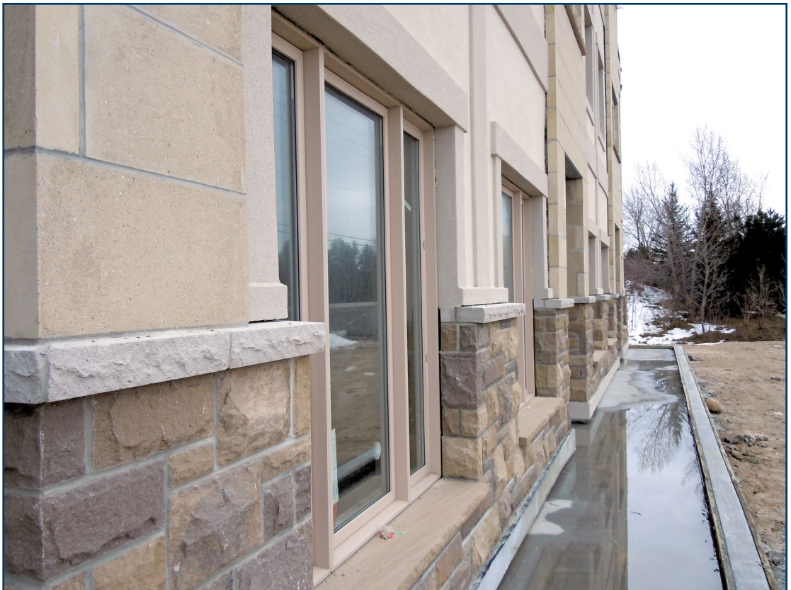
Figure 6 – After the concrete wall is complete, stone and stucco finishes are applied; and the ground around the wall is backfilled up to grade level. (Image courtesy of Roylton Construction.)
