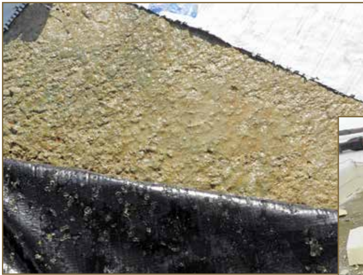
Photo 2 – Moisture between the concrete and self-adhered vapor barrier.
