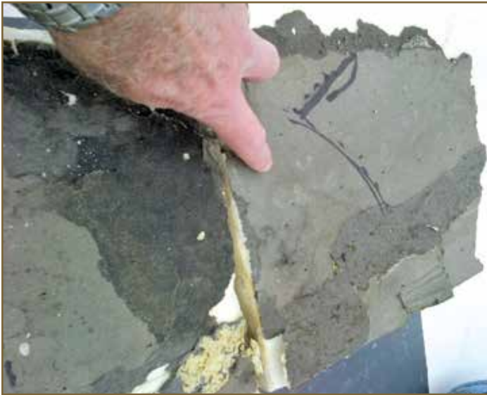
Photo 7 – Moisture underneath the bottom layer of iso.
