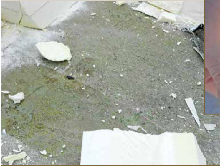
Photo 4 – Moisture on the deck; minimal primer.
