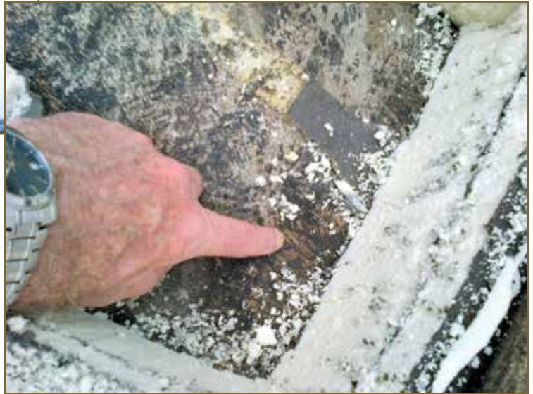
Photo 8 – Moisture on concrete deck.
