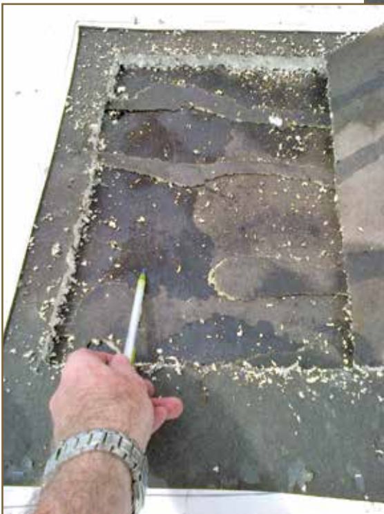
Photo 10 – Moisture between the layers of iso.
