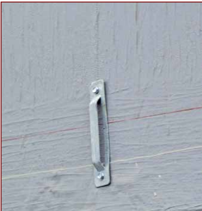
Photo 5 – Steel brick tie not conforming to substrate.
