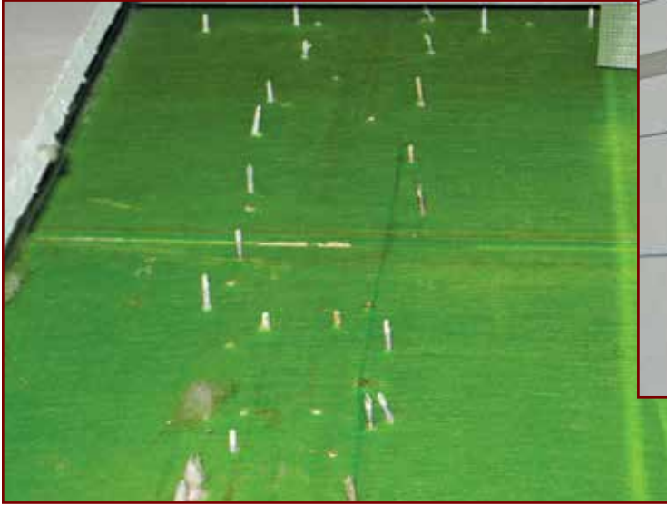
Photo 8 – Fasteners missing studs.
