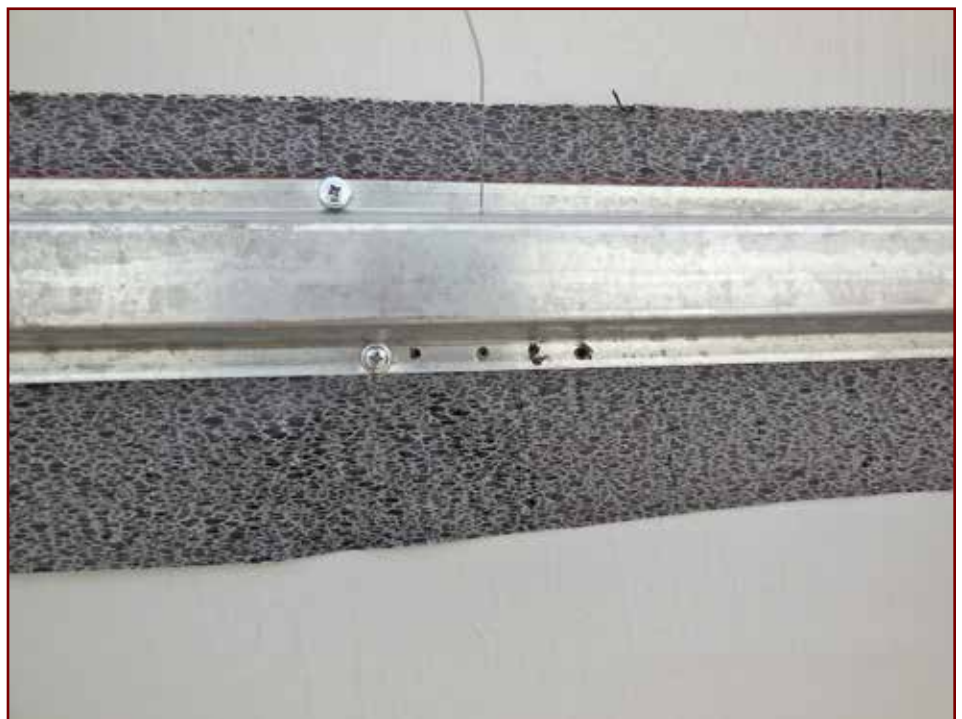
Photo 7 – Multiple fastener holes in flange of hat channel.
