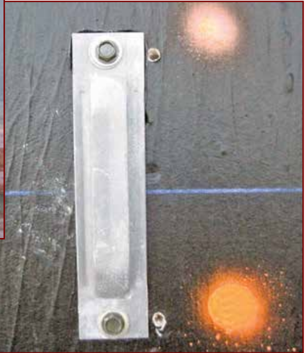
Photo 13 – Holes in WRB adjacent to brick tie.
