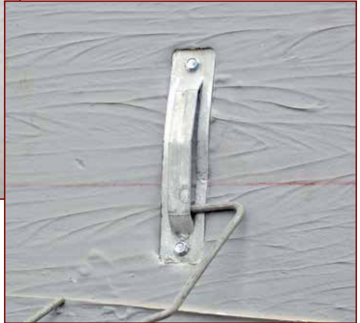
Photo 4 – Brick tie depressed into and damaging WRB.
