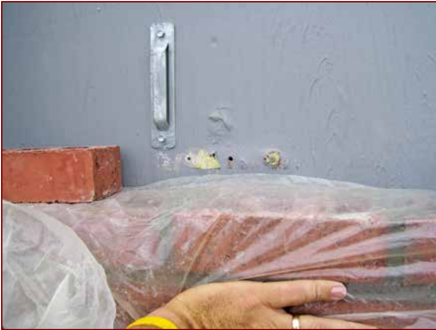
Photo 12 – Multiple holes in WRB.
