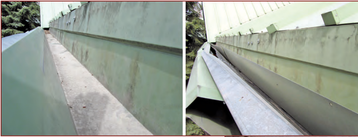
Figure 3 – Integral gutter in place (left) and at beginning of exploratory demolition (right).
