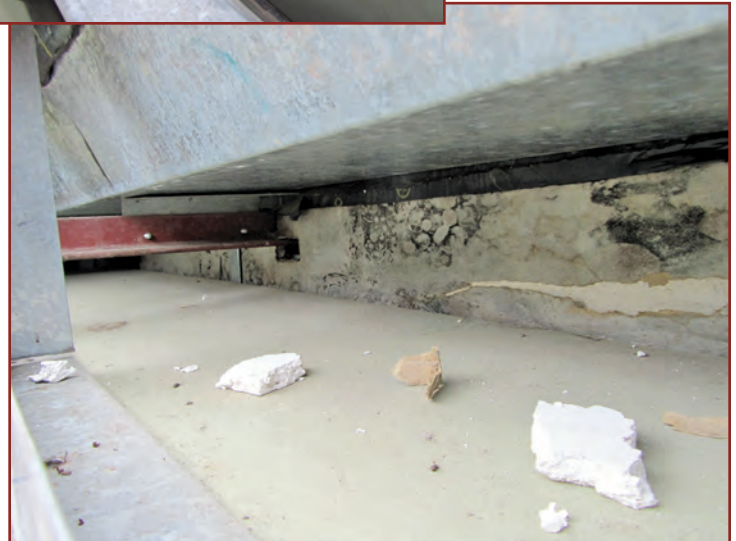
Figure 4 – Mold growth and damage to wall components under and behind integral gutter.
