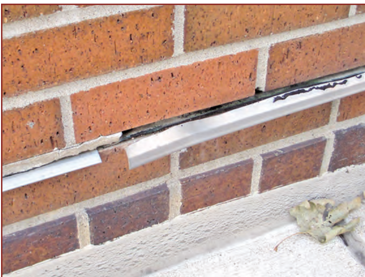
Figure 5 – Fake drip edge inserted into the joint. The contractor must have forgotten to install the stainless steel drip.
