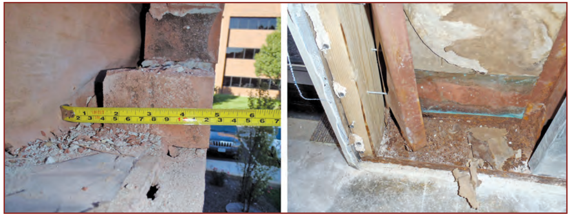
Figure 6 – No drip edge at existing flashing (left) allowed water to saturate the exterior walls (right).
