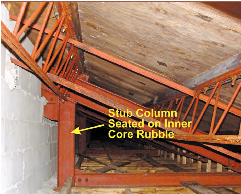
Figure 11 – The hidden-from-view culprit was found to be the location of the steel stub columns.
