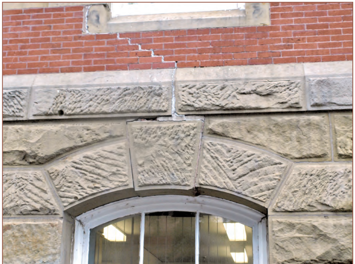
Figure 5 – Example of just one area of cracked masonry, together with a dislodged keystone. Note the failure of the previous repairs.
