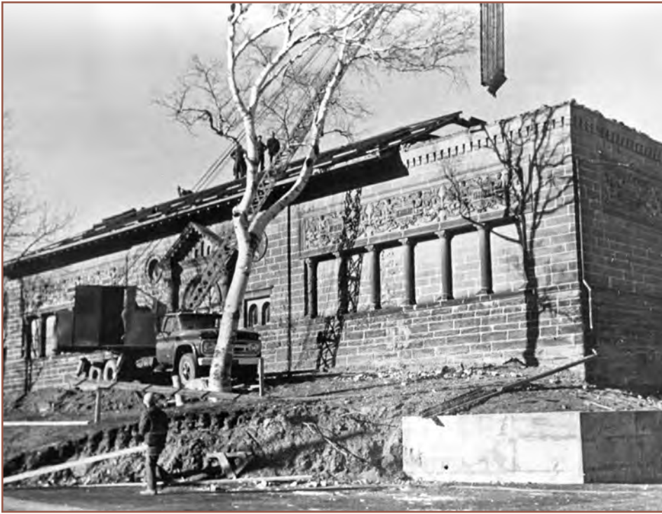
Figure 8 – In 1971, the roof of this building was removed and replaced with a redesigned structural steel superstructure.
