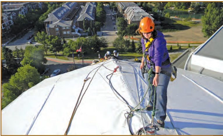
Photo 4 - Mairead Walsh anchors her rope access equipment to a structural member of the Talisman Centre while conducting an investigation of the building's unique tent-like structure.
