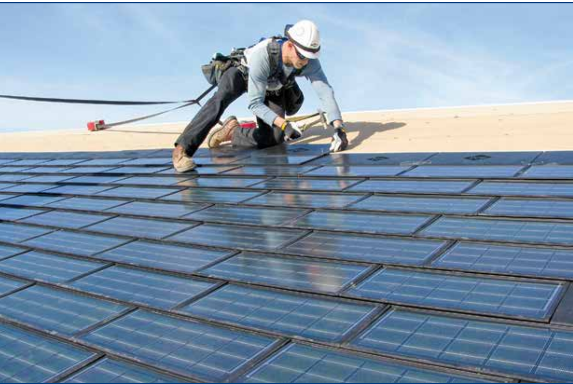
Photo 2 – A technician installs solar shingles on a roof, nailing them just like asphalt shingles (Courtesy of Dow).
