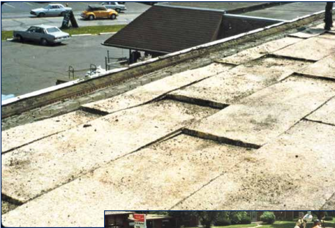
Figures 7 and 8 – When under-insulated or not properly configured with a vapor retarder, sagging or bowing of panels can be experienced over time. On occasion, planks have slumped and fallen out of the array.
