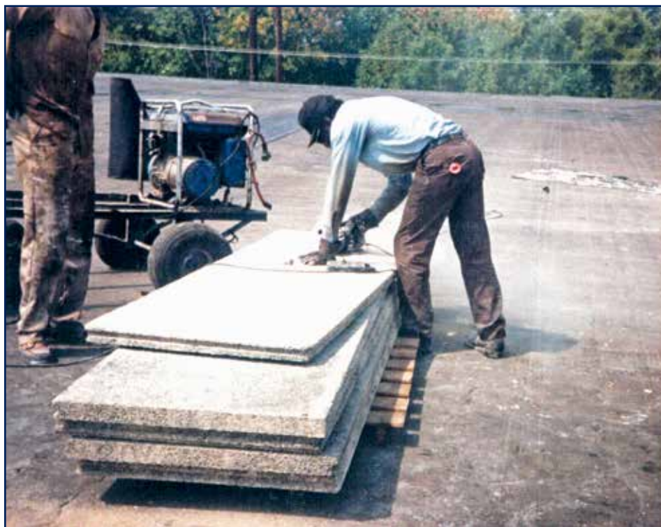
Figure 6 – Planks may need to be field-cut at ridges, hips, valleys, parapets, curbs, and walls; a good circular saw with carbide-tipped blade is usually adequate for this work.
