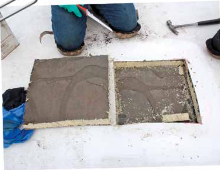
Figure 8 – Removal of insulation at area with several layers. This appeared dry when compared to areas with a single layer. Note removal of top insulation board resulted in cohesive failure of facers.
