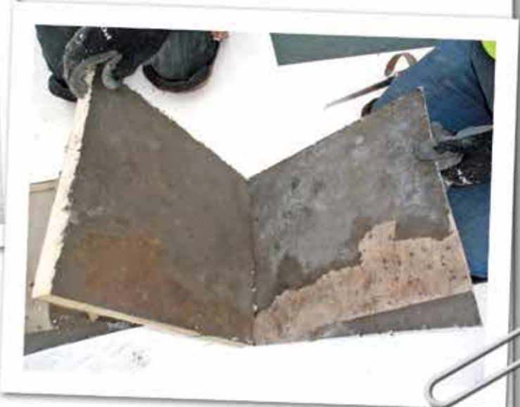
Figure 4 – Mostly (80%+) cohesive failure of facer with remnants of facer on iso board and bottom side of fleece-backed membrane.
