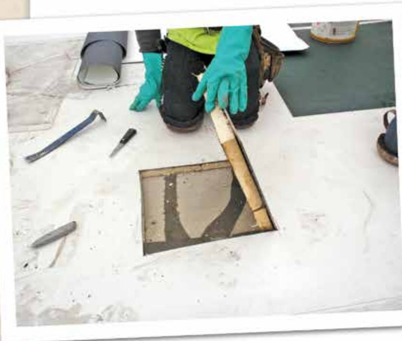
Figure 3 – Cohesive facer failure. Note facer material on adhesive ribbons on deck but no foam core visible.
