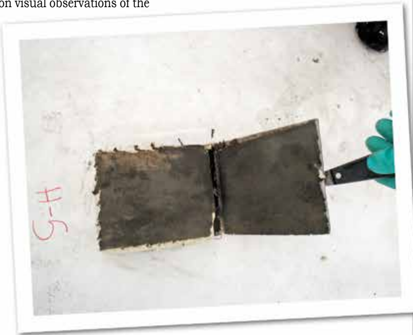
Figure 6 – Cohesive failure of iso board top facer, leaving facer remnants on iso board and fleece-backed membrane.
