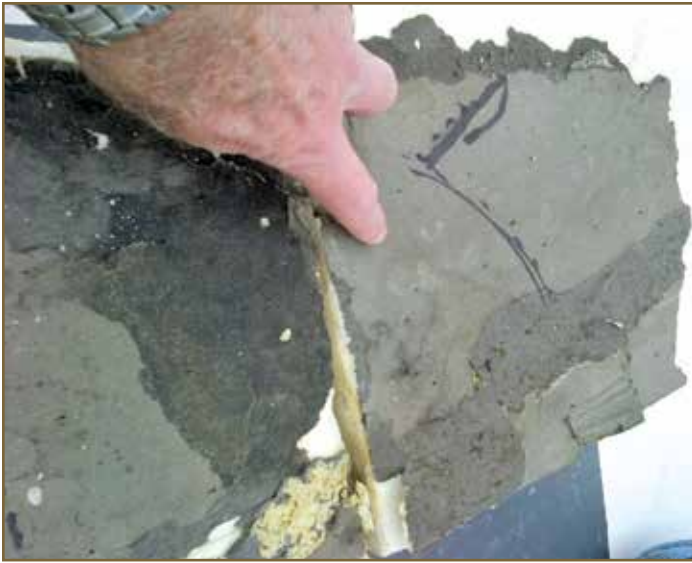
Photo 7 – Moisture underneath the bottom layer of iso.
