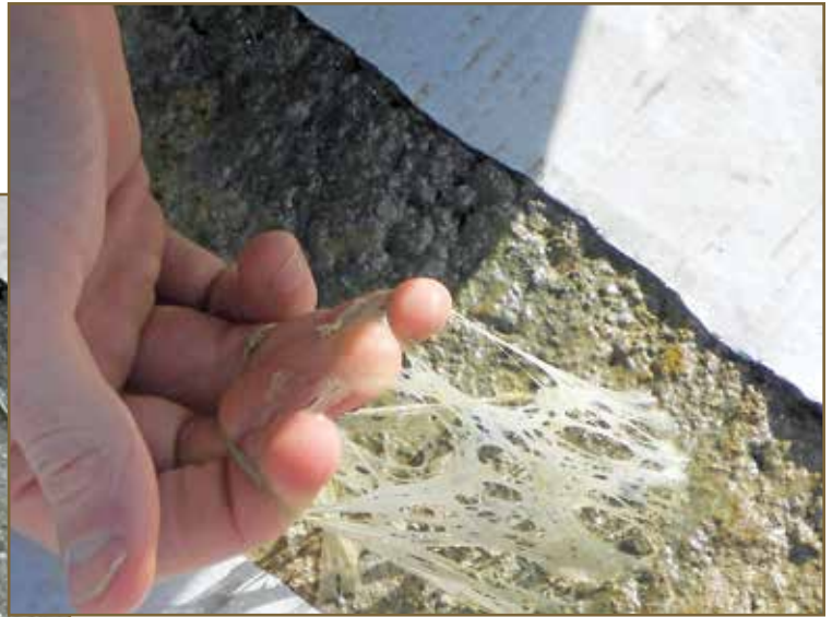
Photo 5 – Primer coming off the concrete deck.
