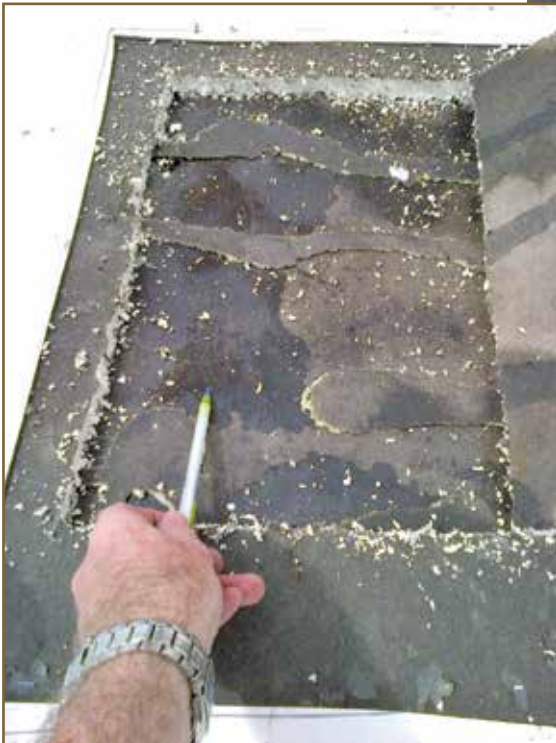
Photo 10 – Moisture between the layers of iso.
