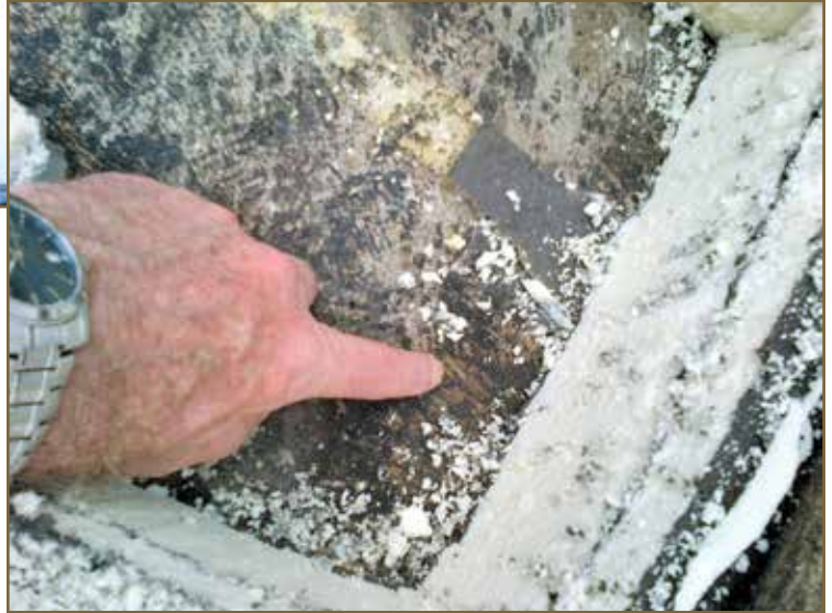
Photo 8 – Moisture on concrete deck.
