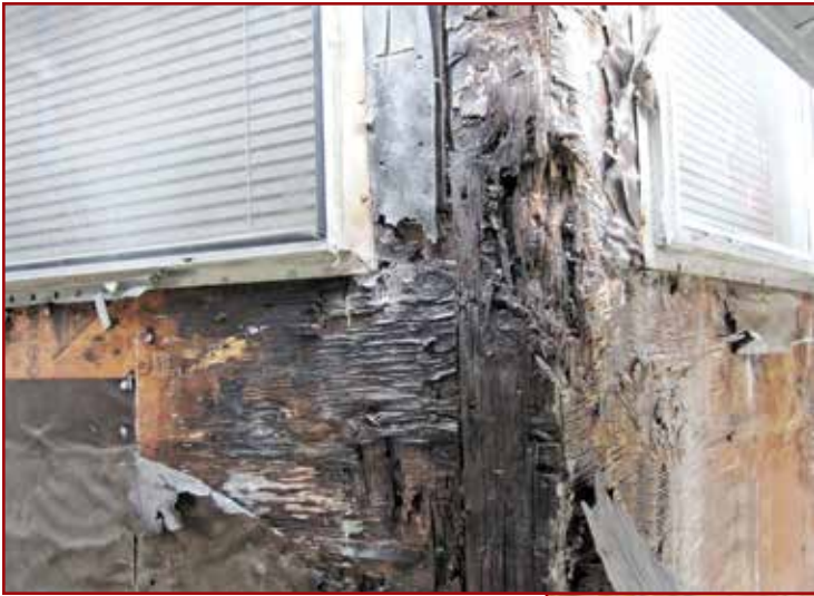
Figure 4 – The leak that got away.
