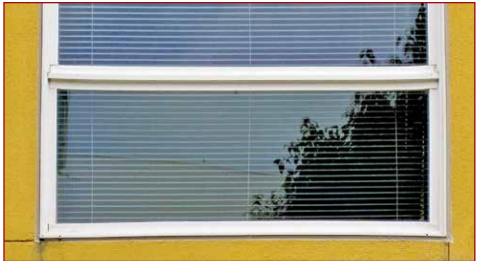
Figure 14 – Deformities in the horizontal mullions caused the glazing beads to exert uneven pressure on the underlying glazing tape. For some windows, glazing beads were cupped sufficiently to channel water into the window assembly, creating another complex pathway for water entry.
