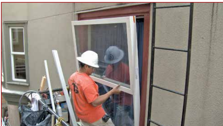
Figure 3 – Want to know why a window leaks? Install windows.
