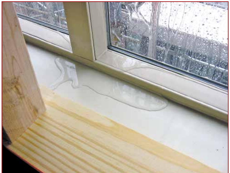
Figure 1 – A puddle beneath the window causes most property owners to suspect windows are leaking. When simple efforts to stop the leakage fail, many surrender to the costly cycle of window replacement.
