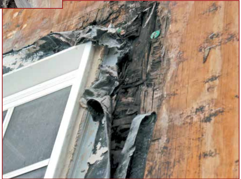
Figure 5 – Perimeter window flashing that performs as an air and vapor barrier prevents drying of water that is trapped or accumulates between the window and the rough opening.
