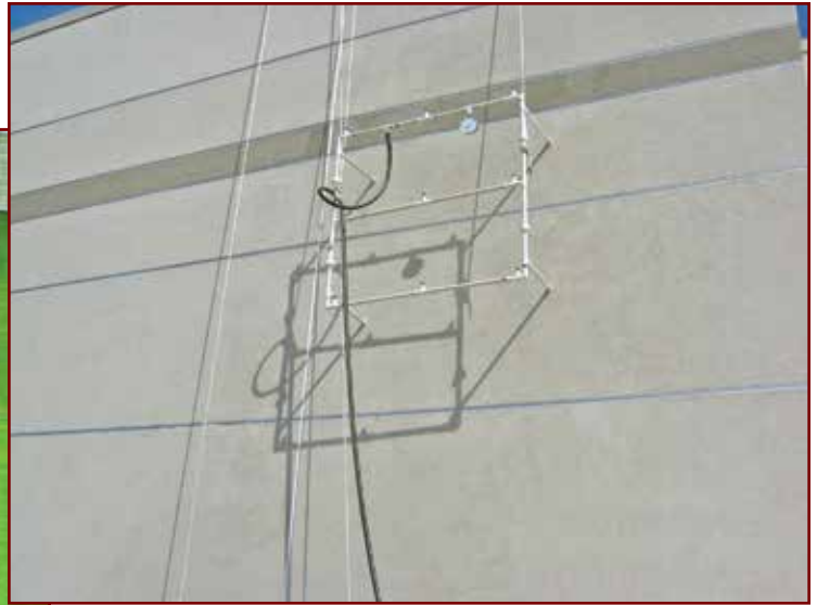
Photo 9 – Calibrated water spray rack on wall.
