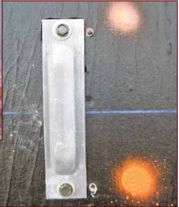
Photo 13 – Holes in WRB adjacent to brick tie.
