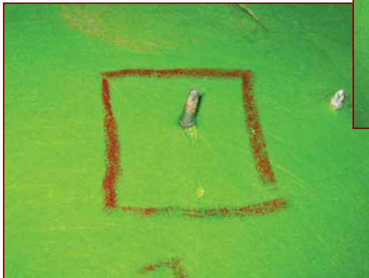
Photo 10 – Water dripping from fastener installed through gypsum sheathing.
