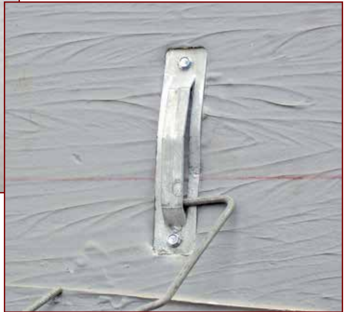
Photo 4 – Brick tie depressed into and damaging WRB.
