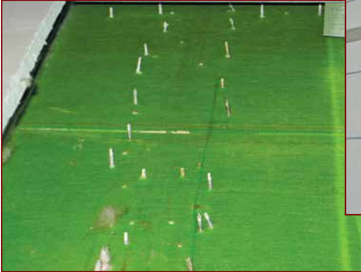
Photo 8 – Fasteners missing studs.
