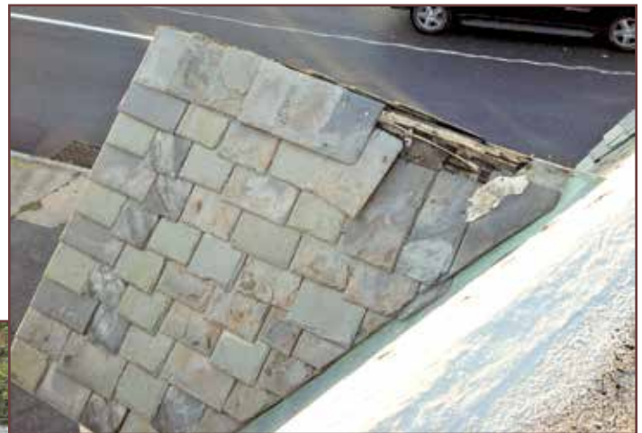
Figure 2 – Areas of slate requiring repair (photo courtesy of SlateSavers).
