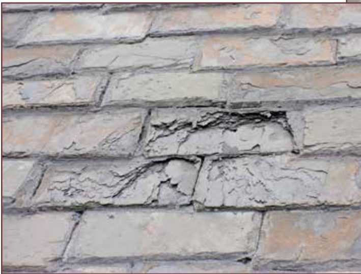
Figure 7 – Close-up of freeze/thaw-damaged slate after grouting.
