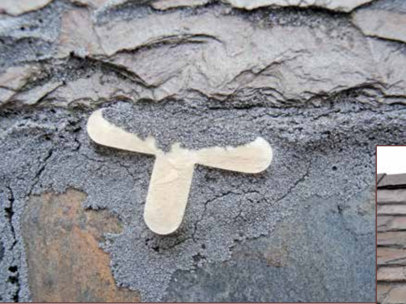
Figure 5 – Slate shim installed low becomes exposed.
