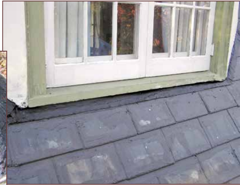
Figure 11 – Exposed slate grout limited to within two inches of slate edges.
