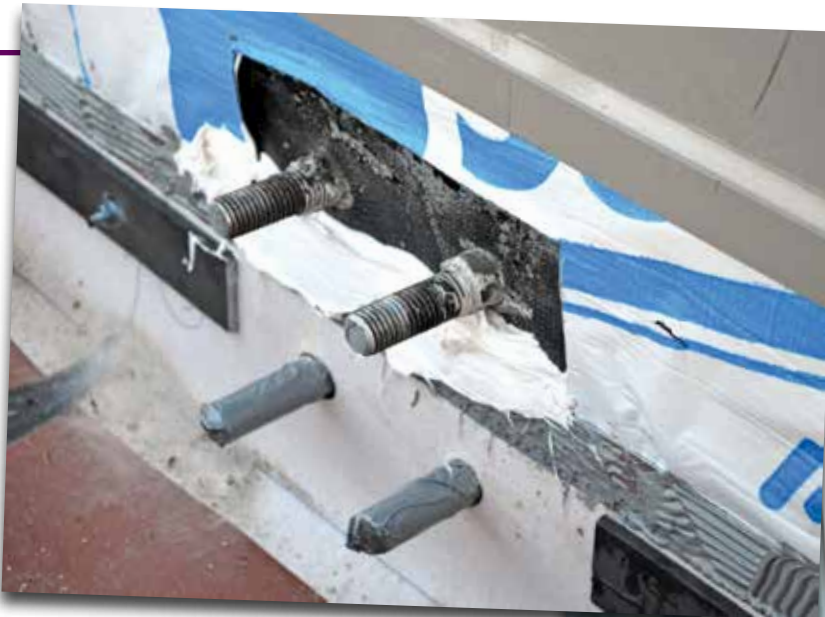
Photo 4 – A close-up showing the adhered and anchored expansion joint at the protection plate supports.
