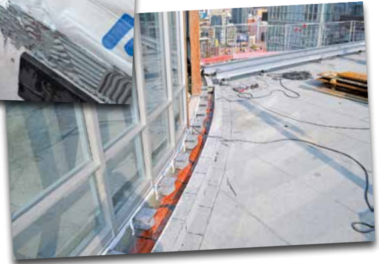
Photo 5 – Completed installation of the west tower joint with the protection plate supports installed.
