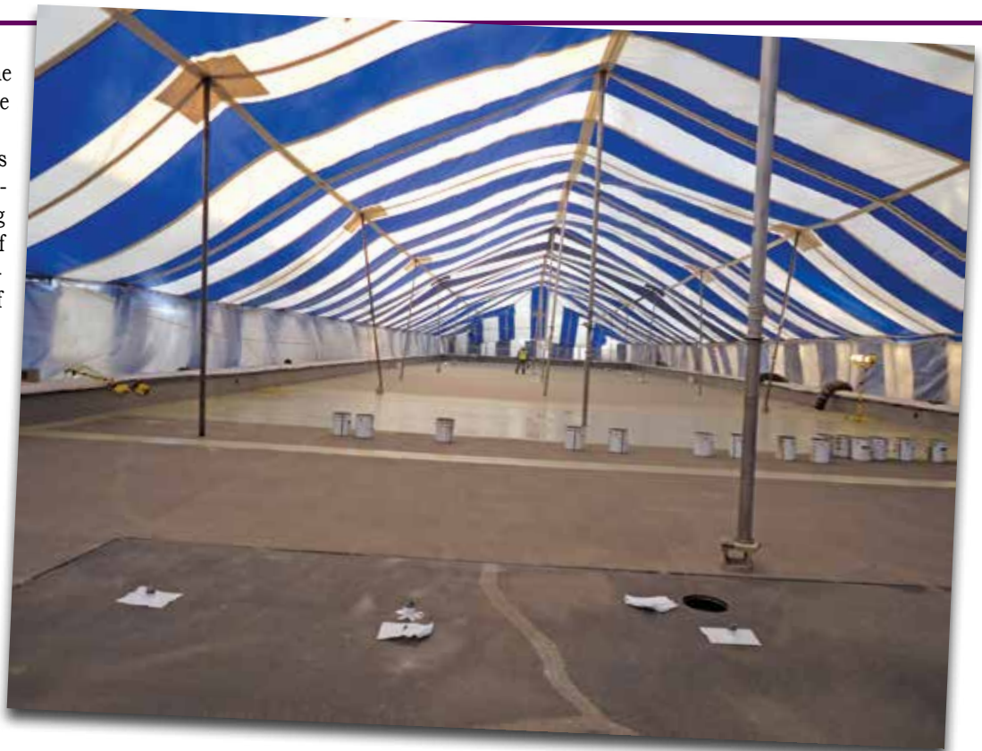
A tent was set up over the entire pool area. The cold liquid-applied reinforced membrane system provides added protection over joints and cracks and around drains and other details. The solvent- and odor-free primer and resin system were important qualities during application.
