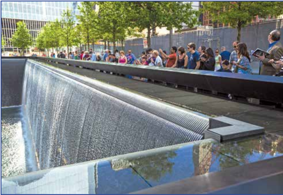
Figure 6 – Troughs and penetrations are hidden from view behind horizontal marble panels. The waterproofing system ties into the stainless steel weirs, which are fully adjustable to control the flow of water into the fountain.
