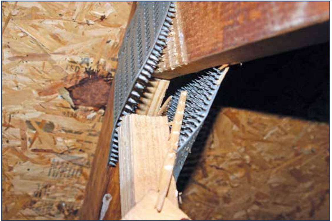
Figure 4 – A sure sign of distress to wood-framed structures is separation of metal plate connectors (gang-nails) in a system of engineered trusses. This is prone to first occur at the king post, and it seems most frequently associated with scissors trusses (i.e., cathedral ceilings having rather long spans). Photo courtesy of Lyle Hogan.
