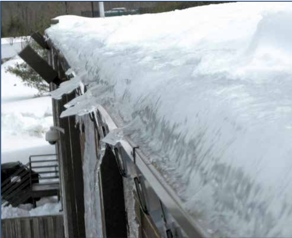
Figure 3 – This low-slope roof has plenty of insulation, but melting and refreezing can pose an issue. Photo courtesy of Richard Wagner.
