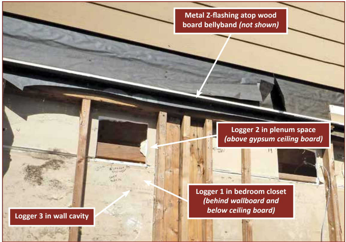
Photo 2 – Parallel wall: At buildings with fiber-cement lap siding, wood board bellybands (not seen in photo) below metal Z-flashings were installed at the rim/plenum transitions.
