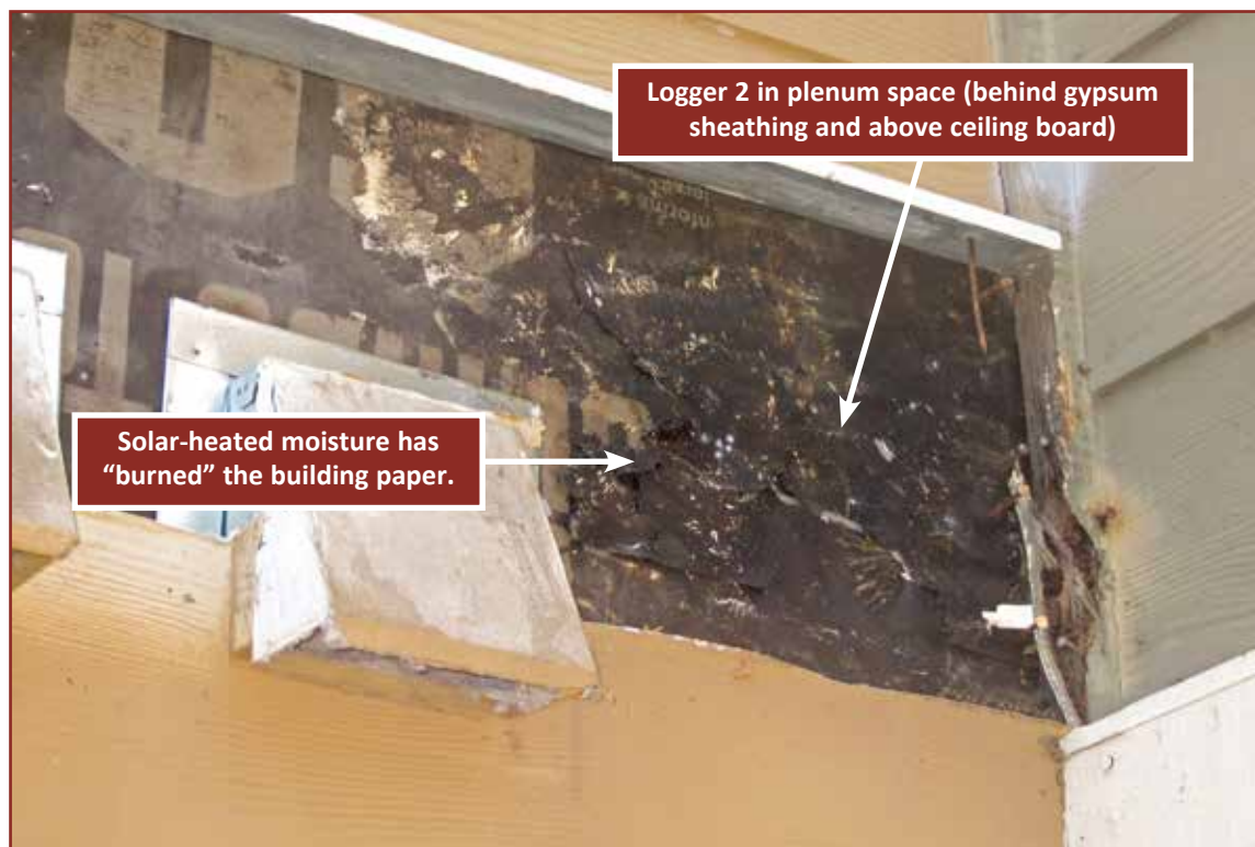
Photo 9 – Rainwater infiltration at nonsealed joints and transitions at metal Z-flashings has led to increased levels of solar-driven moisture migration through the exterior walls (see Graph 9).
