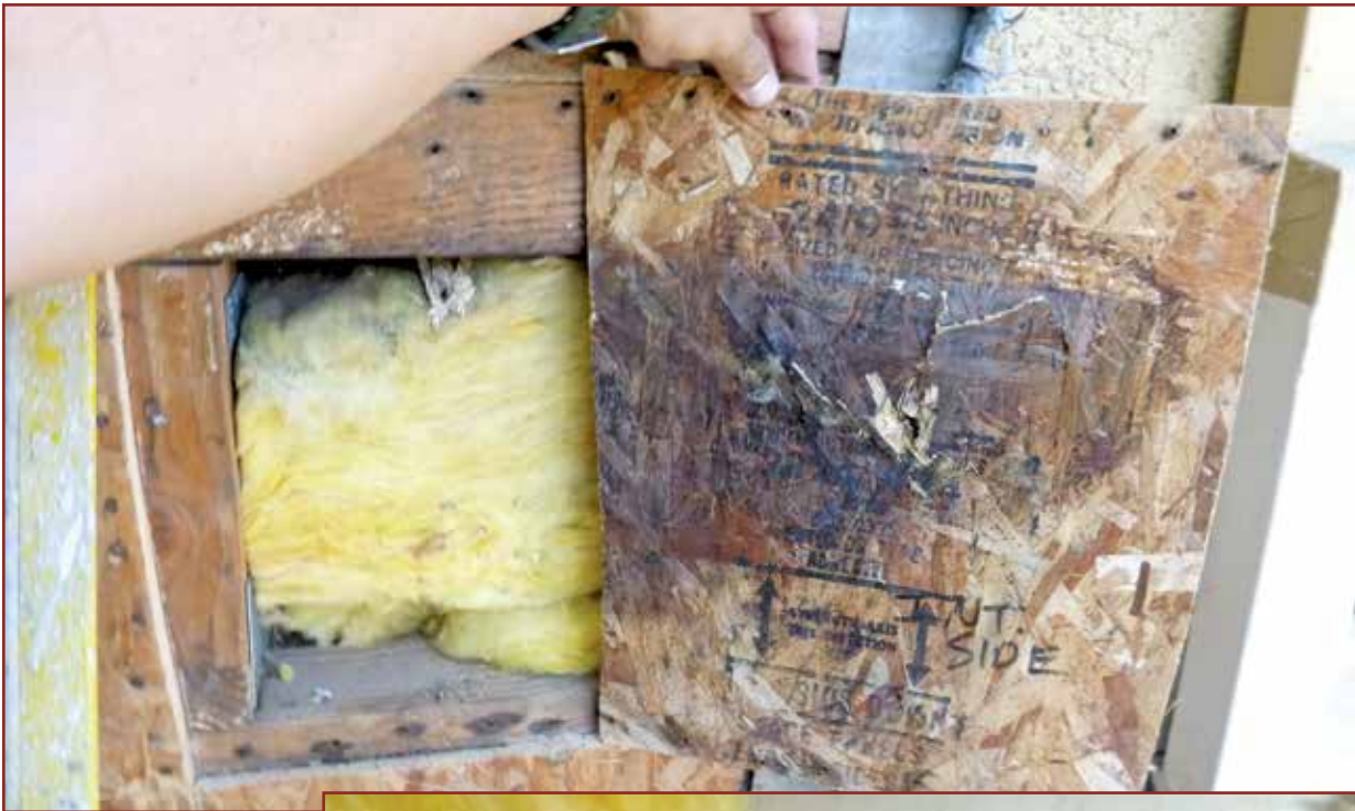
Photo 6 – Perpendicular wall (stucco): No interior envelope was provided at the rim/plenum transition.
