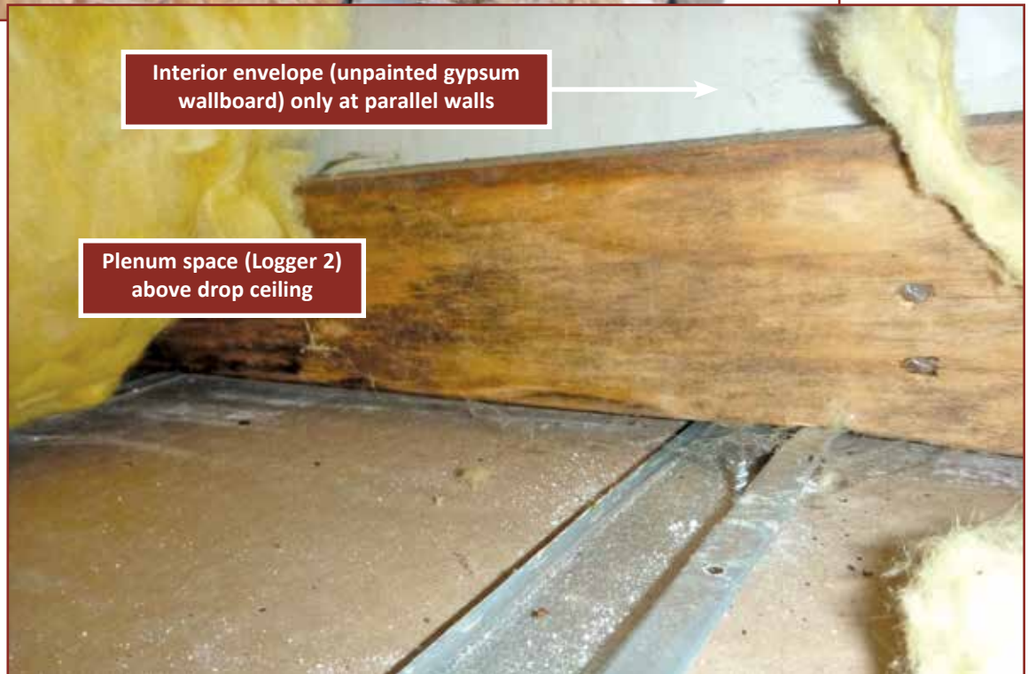
Photo 7 – Typical closet ceiling and interior envelope at parallel wall. At all apartments, the drop ceilings are constructed from gypsum board panels hung from steel resilient channels.
