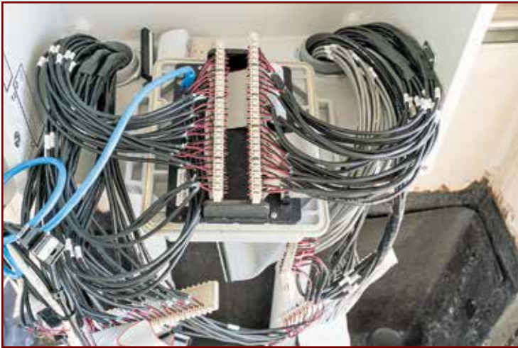
Photo 2 – Wiring and scanning device utilized during construction of a leave-in-place electronic leak detection system.
