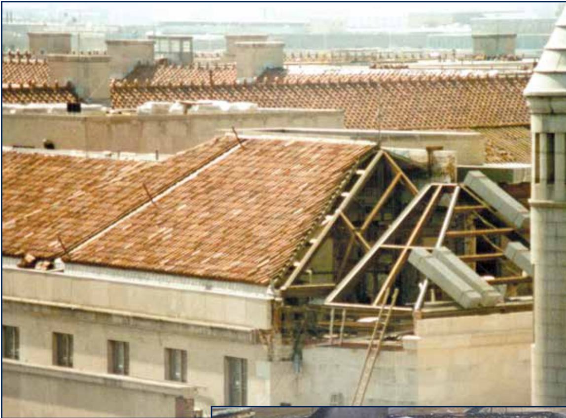
Figure 4 – A precast cementitious plank project in Washington, DC, serving as the substrate for clay tile.
