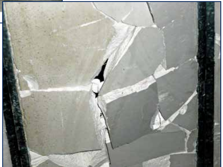
Figure 9 – Without embedded wire reinforcing, this compromised deck would surely have fallen. Note the “white” core, indicating that this is a gypsum product.
