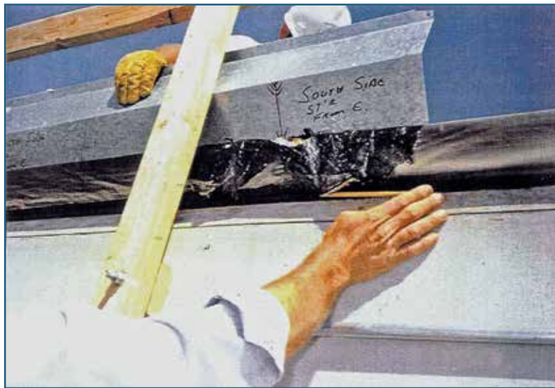
Figure 5 – Torn vapor barrier at the perimeter allowed moist air into the building in the design shown in Figure 4.
