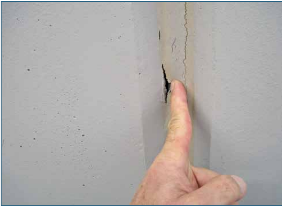
Figure 10 – This sealant joint needs to be replaced as part of reestablishing the air and vapor barrier on the exterior wall of the freezer building.
