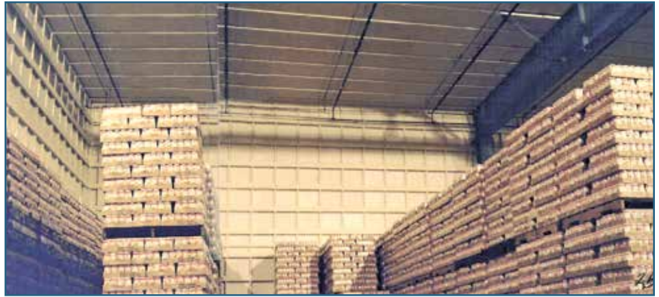
Figure 3 – Fiberglass insulation held in place with wood frame/grid in frozen-juice plant.
