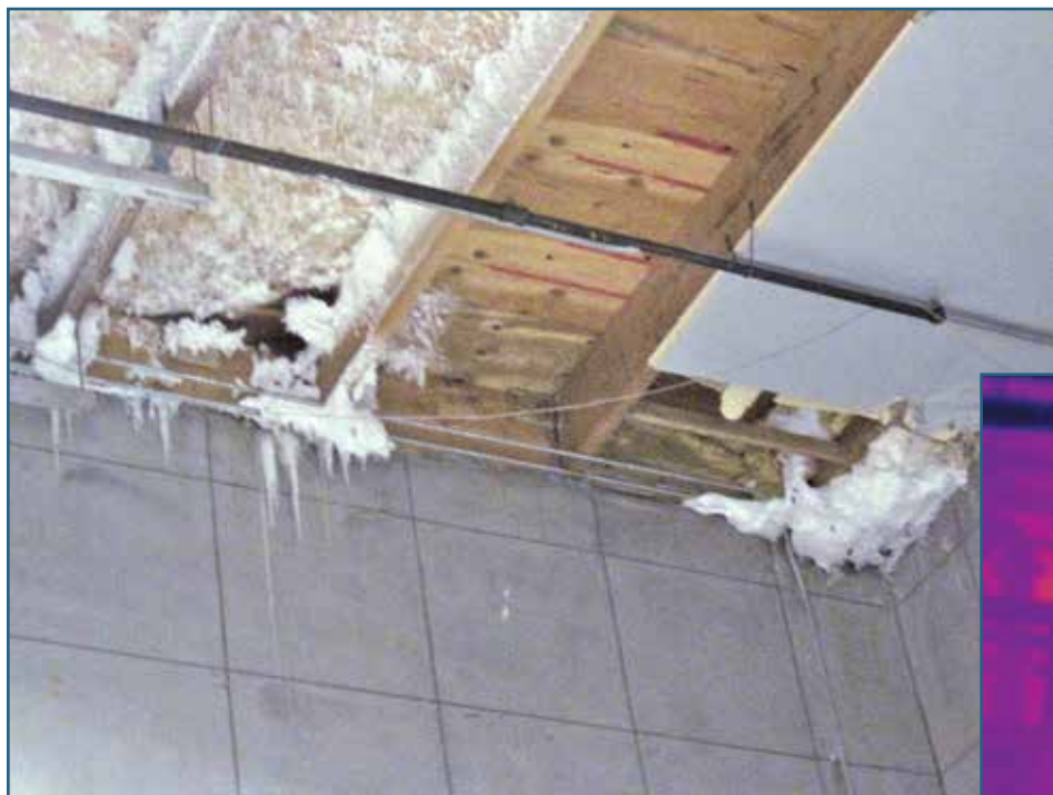
Figure 6 – Icicles extending down below the roof-to-wall joint due to air leakage from the exterior.
