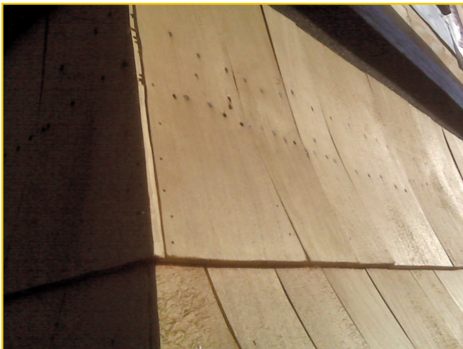
Photo 8 – Far too many fasteners on this application.
