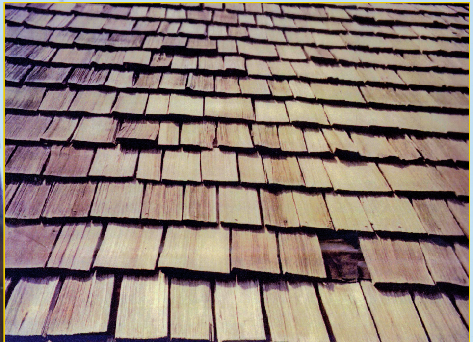
Photo 1 – Rot-felted application where felt paper has started to degrade following UV exposure.
