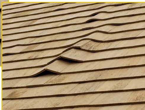
Photo 14 – Buckling due to improper keyway spacing.
