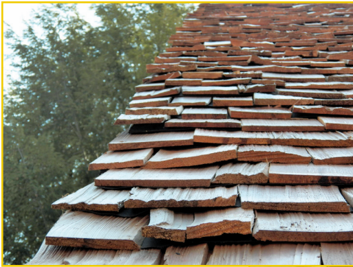
Photo 11 – This photo shows an improper application. Some of the issues we see here are excessive flat-grain, off-grade material, lack of keyways, and uneven courses.
