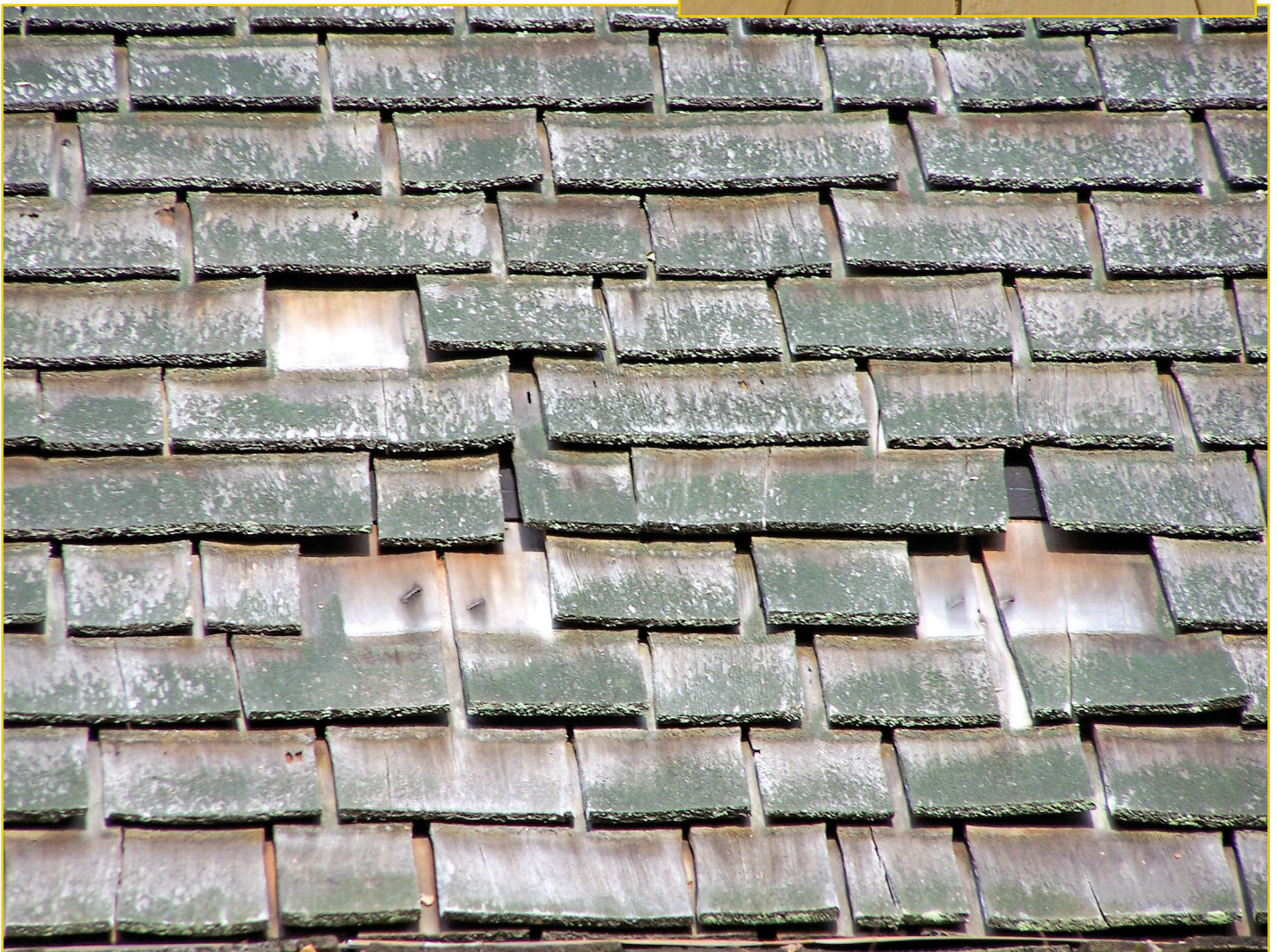
Photo 6 – Fastener issues causing roof failure.
