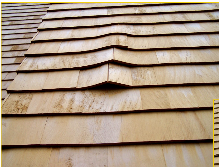
Photo 13 – Buckling due to improper keyway spacing.
