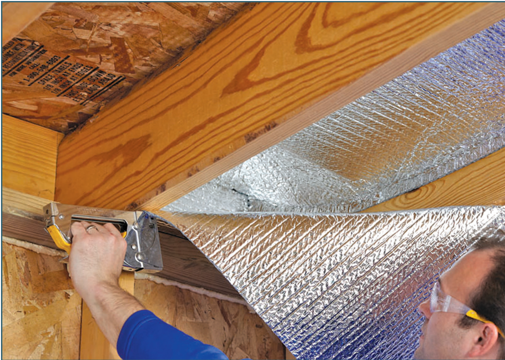
Figure 4 – Reflective insulation installation of a double-layer R-21 to a floor joist in crawl space.
