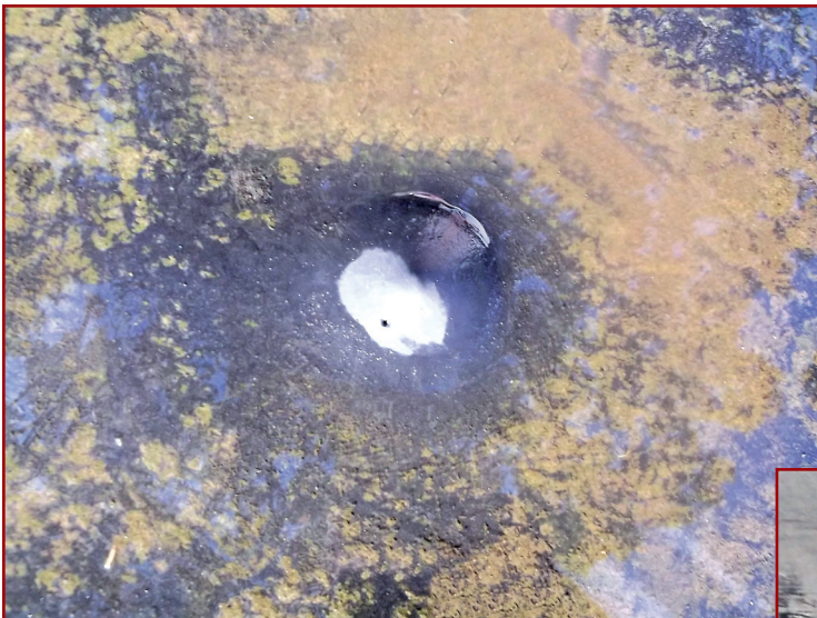
Figure 6 – Although in near proximity, the tiny holes encountered here were not punctures from the nearby fastener head. The “tented” fasteners, however, may well provide the necessary underside space accommodation for the guilty insect to make the openings.
