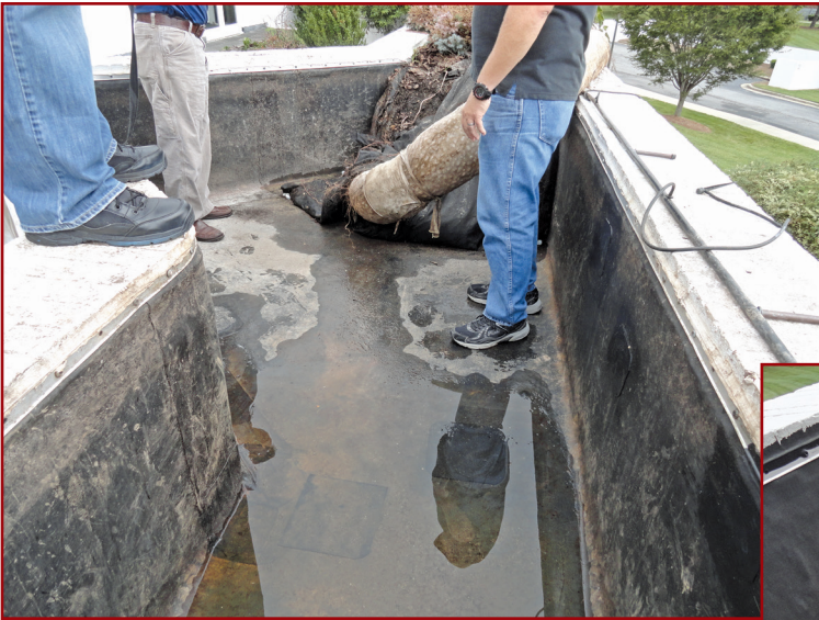
Figure 3A – This vessel incurred substantial cost, requiring removal of overburden where insect boreholes were eventually located.
