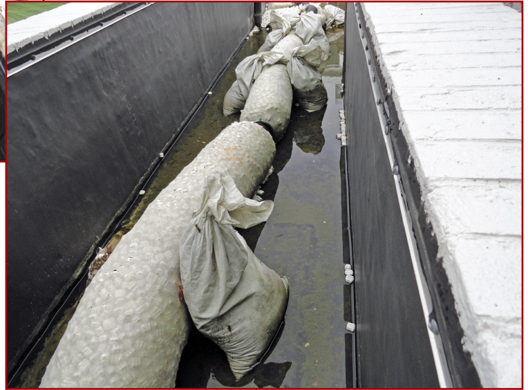
Figure 3B – This vessel was similarly lined with EPDM (same contract) but never received mulch, soil fill, or plantings; leaks have not occurred below it in the years since installation.
