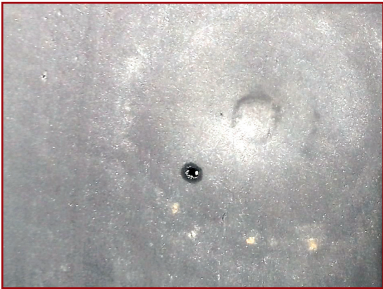
Figure 8 – While the openings are quite small, prolonged ponding can exacerbate the tendency for any breach to admit a substantial amount of water.
