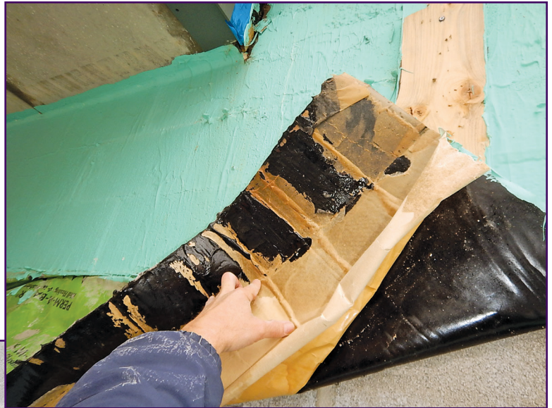
Figure 3 – Two months after seeing Figure 2, note the same TWF with intermittent loss of release paper and exposure to the elements, leaving self-adhesive or “sticky” side compromised to the extent that failure will occur.
