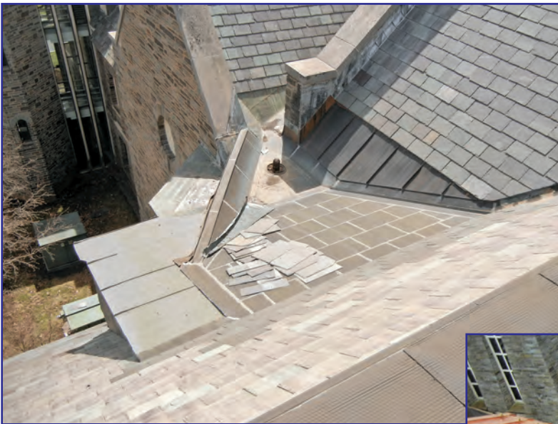
Figure 13 – Drainage basin around the corbelled dormer prior to the project.
