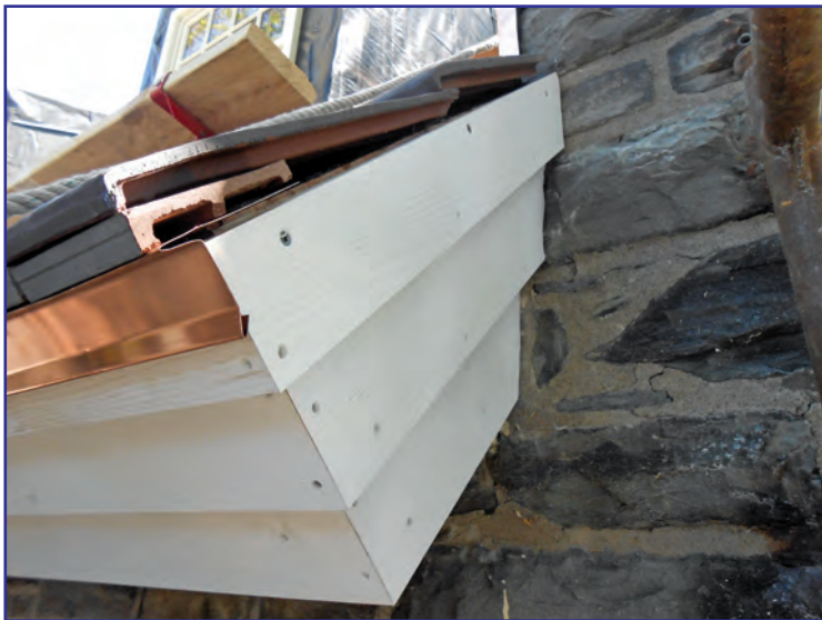
Figure 8 – The rake-end condition of the interlocking clay tile assembly, prior to completion.
