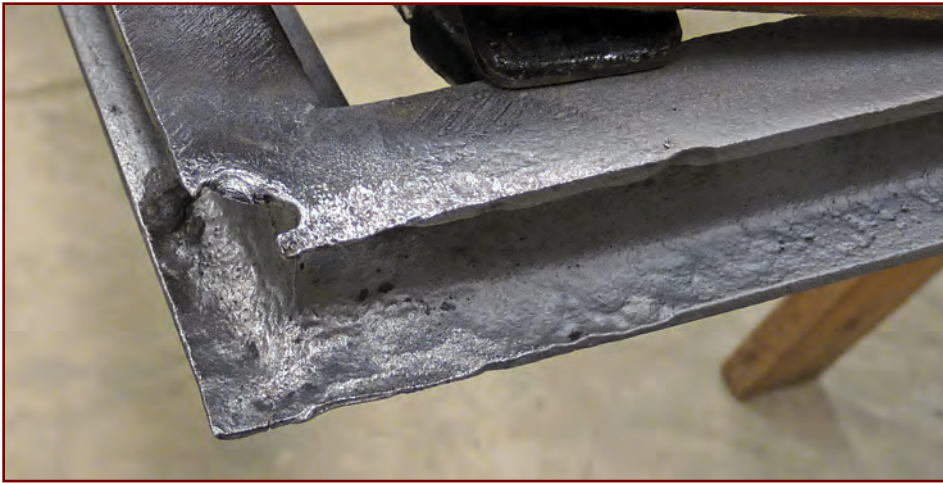
Figure 7 – Example of severe corrosion of the steel sash.
