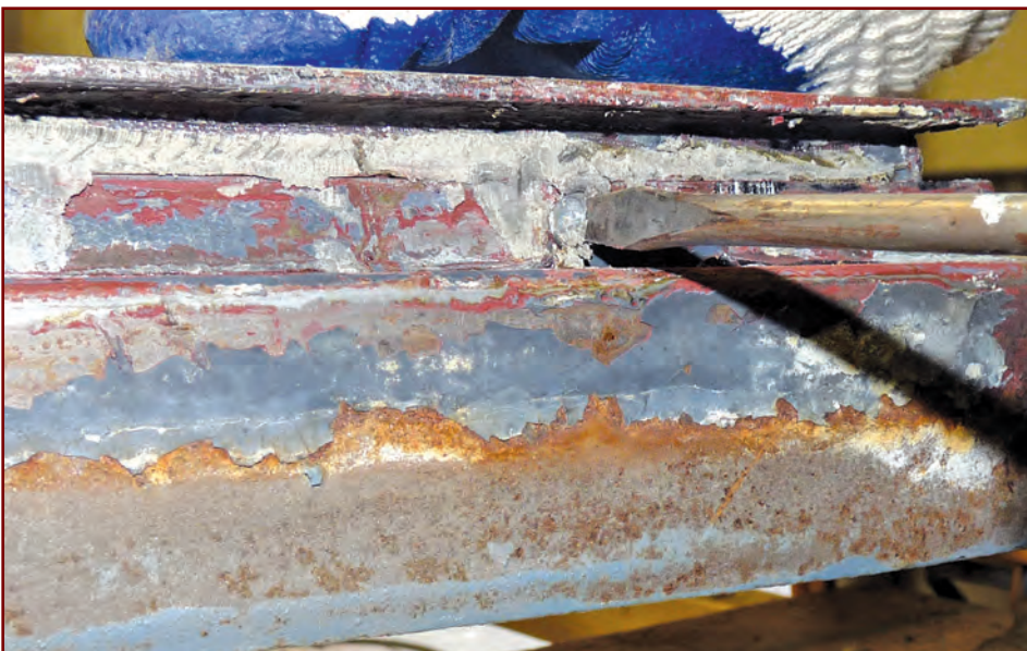
Figure 6 – Example of moderate corrosion of the steel sash.
