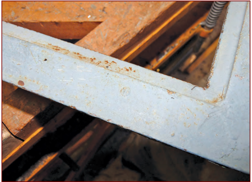
Figure 5 – Example of minor corrosion of the steel sash.
