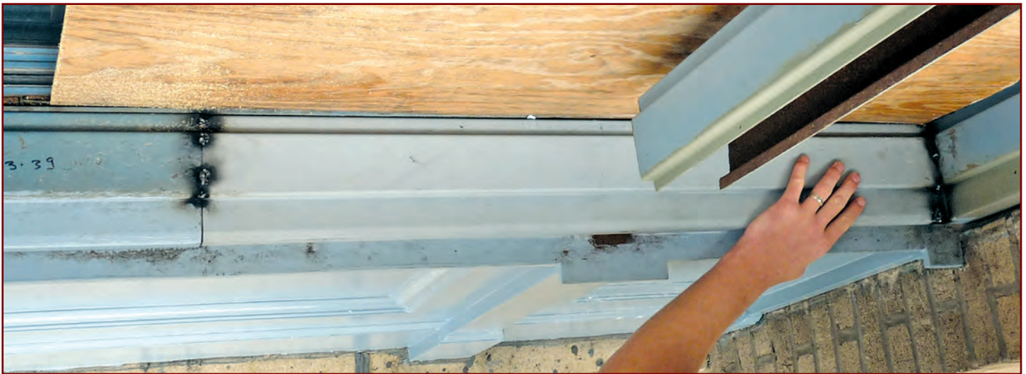
Figure 11 – Sub-frame repair in process. Replacement section tack-welded in. There is a steel backing plate that spans the joint. Welds will be made continuous along the joint and ground flat to the profile. Where required, epoxy patch material will be added.
