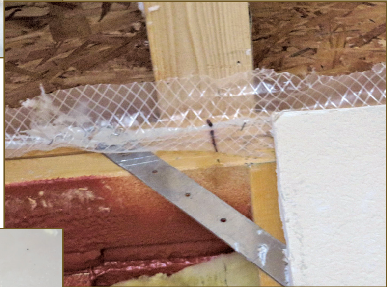
Figure 3 – Vapor retarder bypass at partition and party walls.
