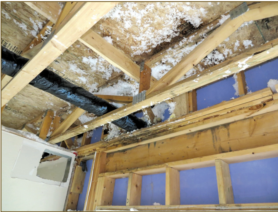
Figure 6 – Leaky dryer and bathroom vent ducts in truss space.
