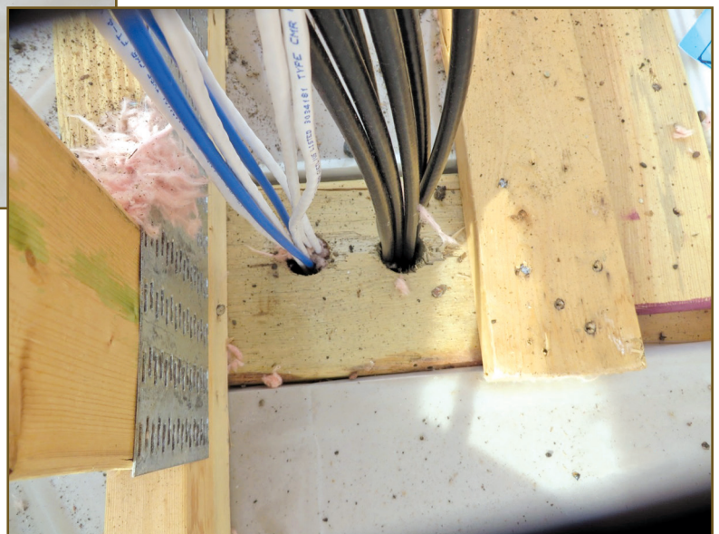
Figure 5 – Vapor retarder bypass through top plate of partition wall.
