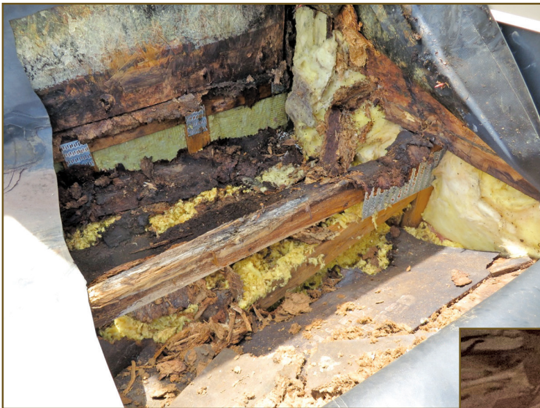
Figure 2 – Rotted deck collapsed into truss space revealing rotted top chord of truss and corroded tie plates.
