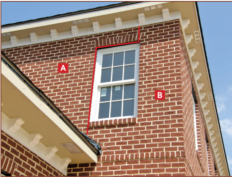
Figure 6 – The red line denotes location of a crack due to lack of isolation joint between elevation segments A and B, which have different bearing conditions. Segment A bears on steel, and segment B bears on the foundation below.
