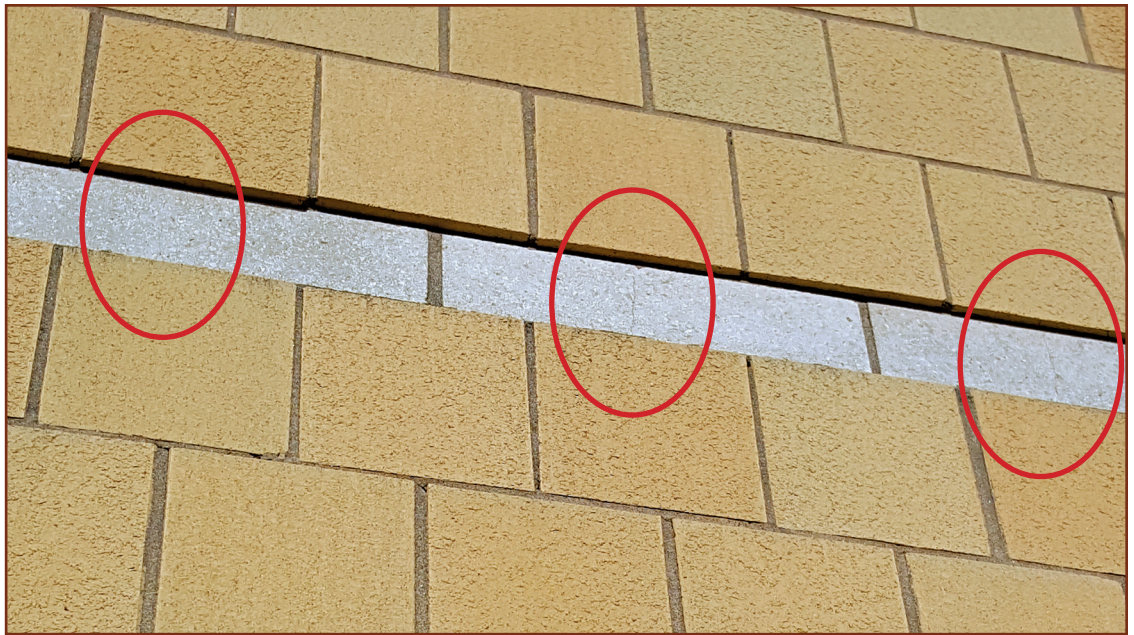
Figure 8 – Approximately 80% of all CMU units are cracked in the accent bands on this large hospital project because of differential movement of the shrinking CMU band bonded to large expanses of clay brick veneer.
