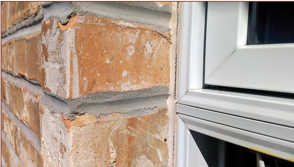
Figure 9 – This sealant joint prematurely failed because there was no room to install a backer rod for a properly formed sealant joint. Designers should draw and dimension a gap on all four sides of windows.
