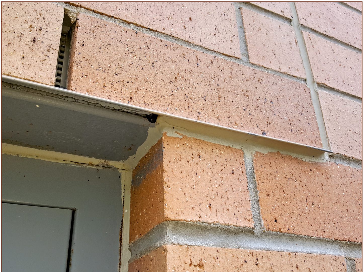
Figure 7 – Vertical movement joint properly located at the end of the beam bottom plate that supports the clay brick veneer at the door opening. Sealant properly installed under drip edge to prevent wind-driven rain penetration.
