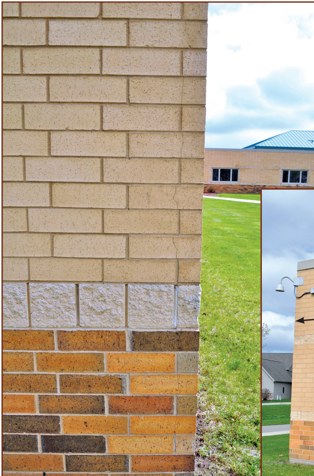
Figure 3B – Crack developed at the corner because veneer movement joints were spaced too far away from the corner on both sides.
