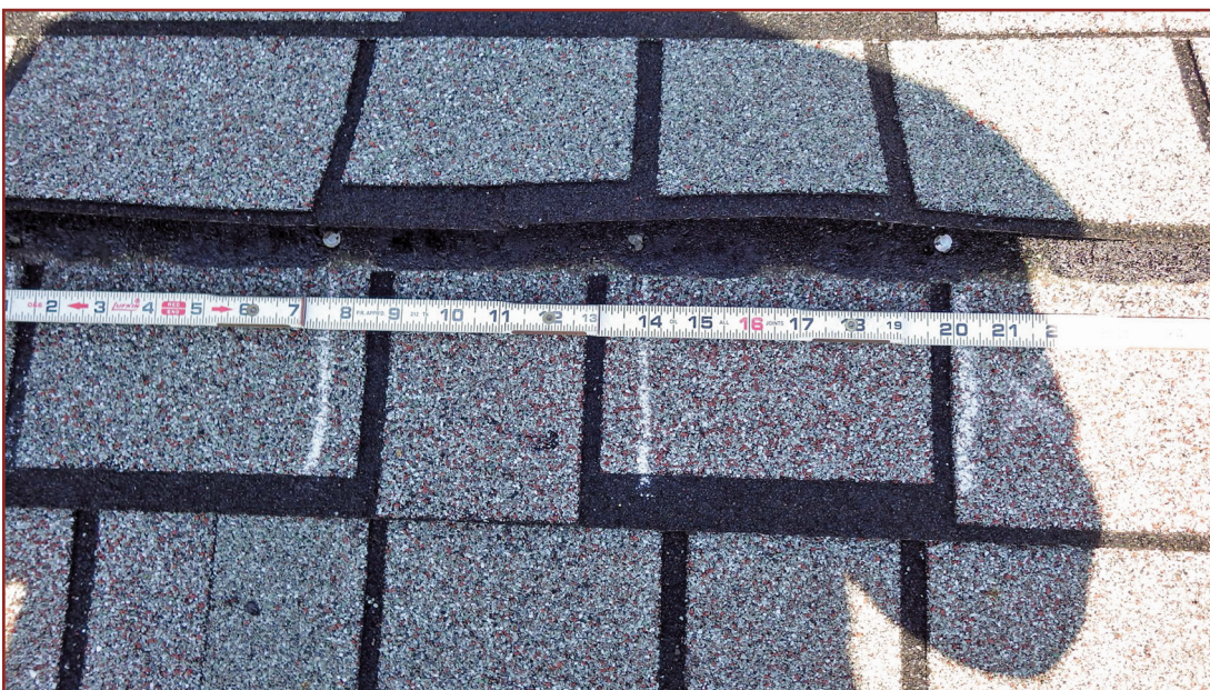
Figure 4 – Forensic investigation of shingle installation documenting fastener placement.
