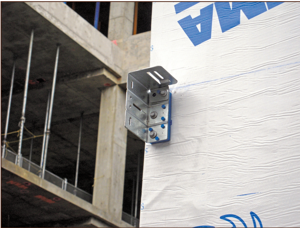
Figure 6 – Installation of the thermal clip used in Case Study Two over self-adhered membrane.
