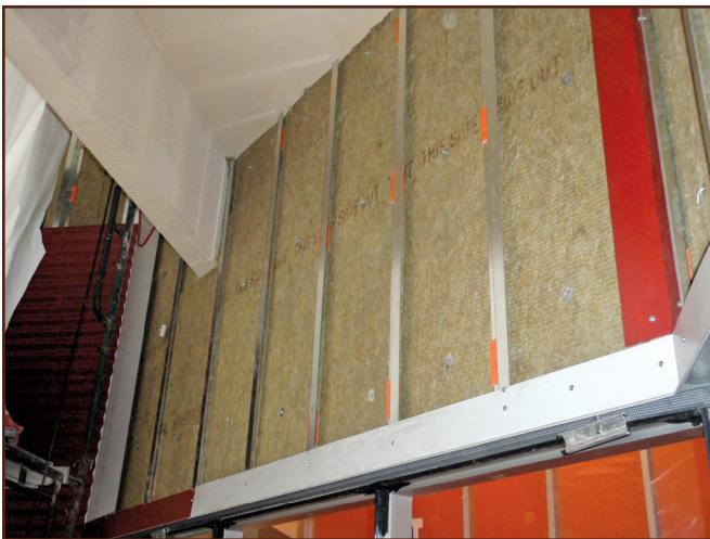
Figure 4 – A layer of exterior insulation behind the Z-girts was secured to the fiberglass thermal clips of the building in Case Study One.
