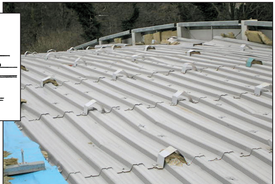
Figure 3 – Close-up of wind damage zone showing detached top hat rails and distorted saddles.
