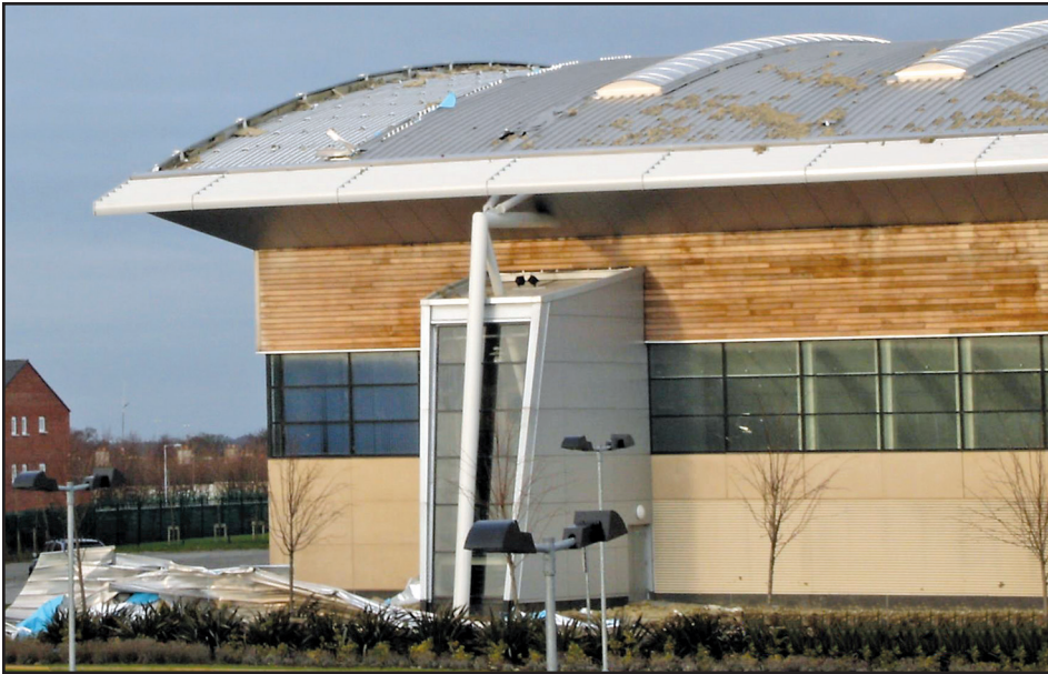
Figure 2 – Detachment of aluminum standing seam roofing from windward verge of the Competition Pool.
