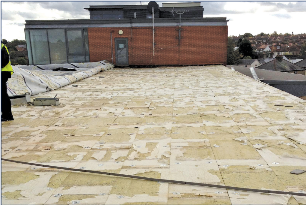
Figure 5 – Second-floor roof membrane rolled back from western edge.
