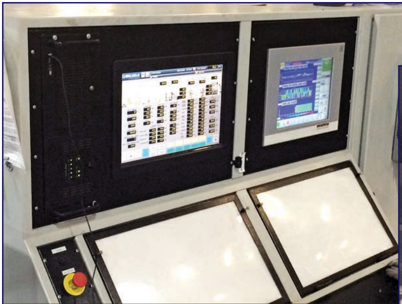
Figure 3 – Computer-integrated controls for process control.
