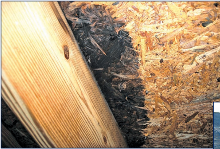
Figure 9 – OSB is rather intolerant of moisture exposure, so ongoing leakage is sure to cause problems. Remember that board edges can expand by up to 15%, especially if they are cut edges.
