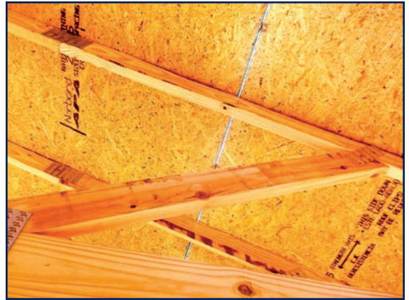
Figure 8 – As suggested by APA, a 1/8-in. gap should be provided along all sides. Here the deliberate spacing is shown.
