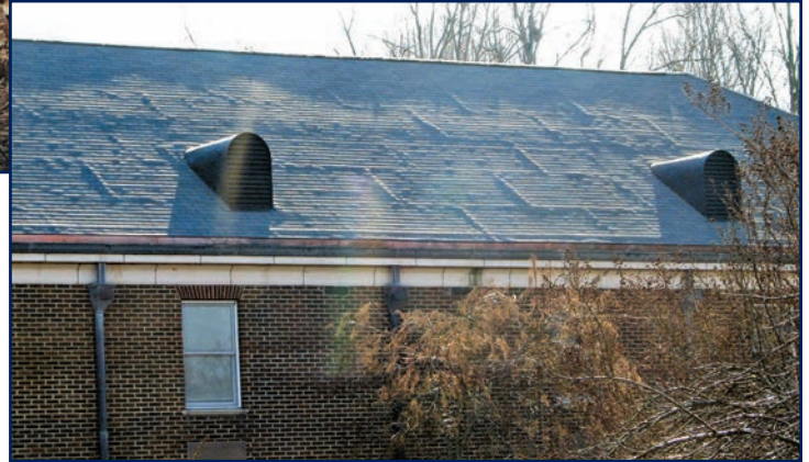
Figure 10 – Deck buckling usually stems from substandard ventilation, improper attachment along panel edges, failure to provide space between sheathing panels, or some combination of these. With sufficient attic ventilation, proper spacing of sheathing, correct attachment, and correct span/thickness relationships, virtually all surface undulations can be avoided.
