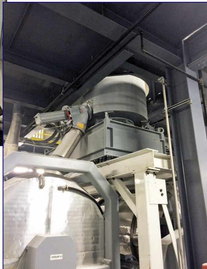
Figure 4 – High-speed blender and cooler.
