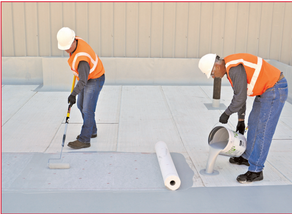
Figure 7 – Trained crews can apply PMMA roof membrane systems very efficiently. This application efficiency, together with PMMA’s fast cure times, allows advantageous scheduling options.
