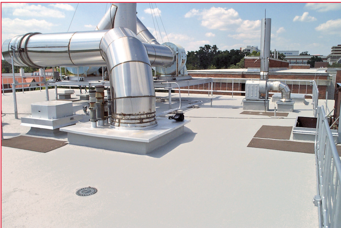
Figure 4 – PMMA systems provided an efficient application solution for the crowded roof of this facility.
