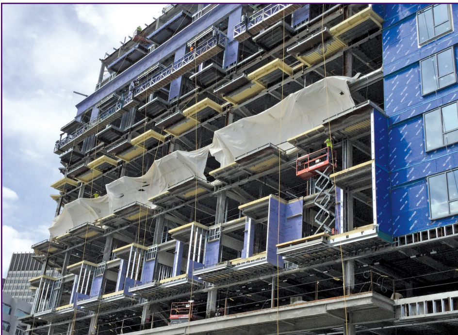
Figure 10 – AFC applied to concrete balconies of a residential tower in Boston, MA.
