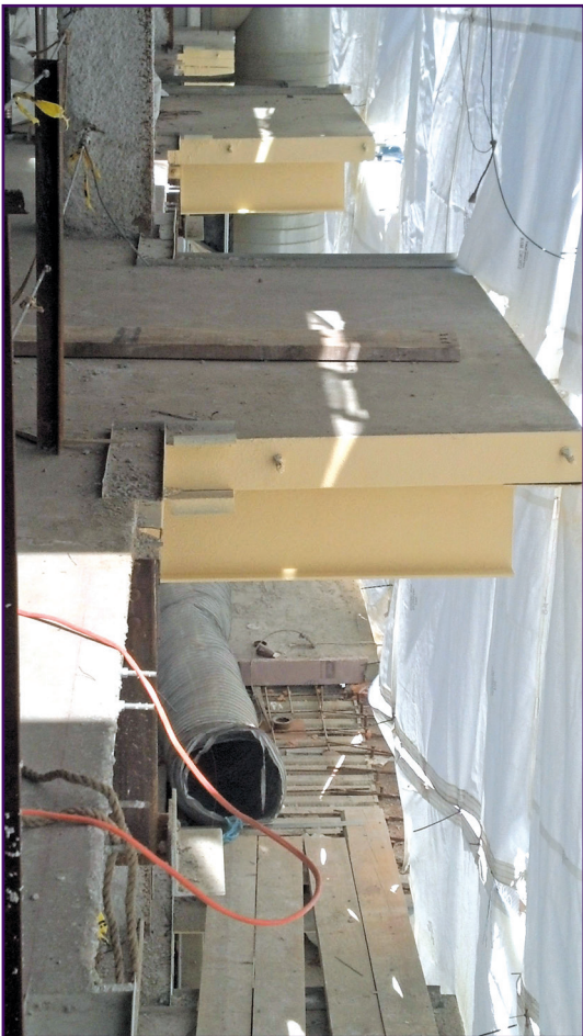
Figure 8 – Concrete balconies coated with 100 mils of AFC beneath pavers (ICON Architects, Righter Group.)
