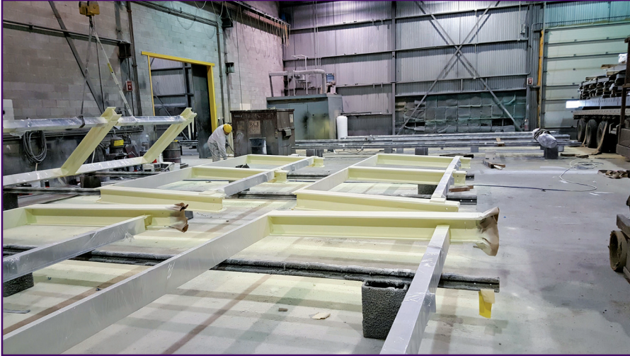
Figure 6 – Shop-applied AFC fluid-applied thermal break coating applied to outriggers on 20-story mixed-use project.
