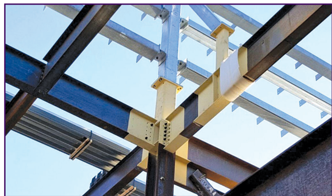
Figure 5 – AFC used in conjunction with bolted AD moment connections (blocked out) and touched up in field.
