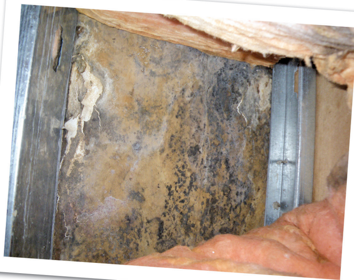
Figure 2 – Typical deterioration of gypsum sheathing to which the EIFS was adhered and corrosion on the steel studs.
