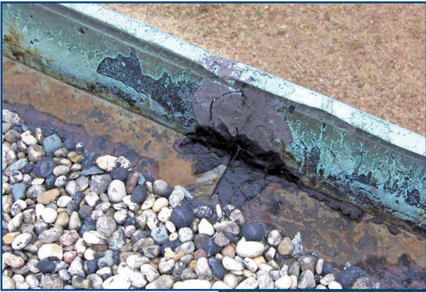
Figure 2 – Improper patch to existing copper gutter.
