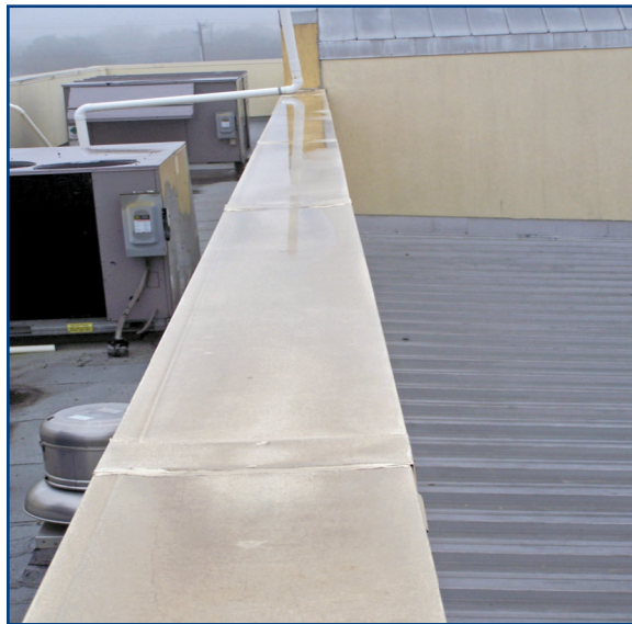
Figure 6 – Coping with concave profile retaining water.
