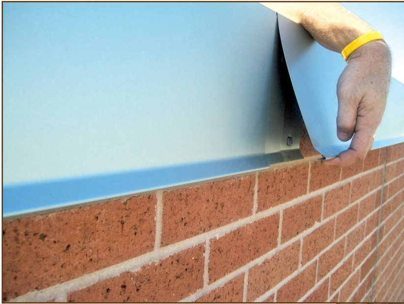
Figure 15 – Fascia of coping not engaged to cleat.
