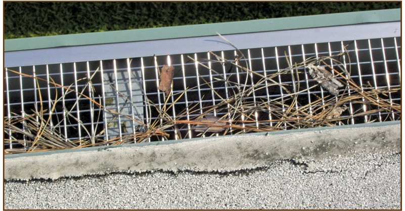
Figure 8 – Urethane sealant disbonded along edge of cap sheet.
