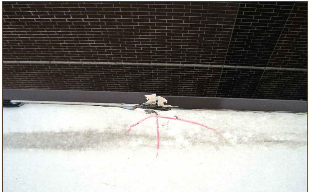
Figure 12 – Deteriorated sealant at joint in metal.
