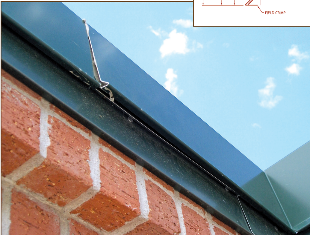
Figure 14 – Metal snap-on fascia not engaged to cleat.
