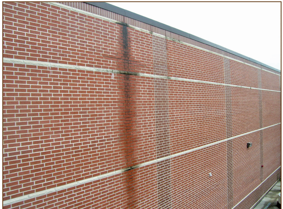
Figure 11 – Biological growth on brick from leakage at joint in metal edge.
