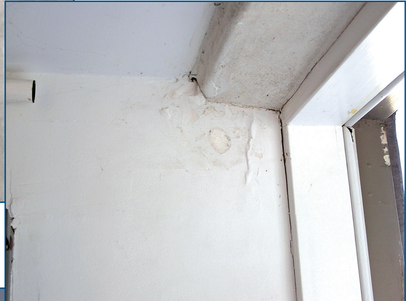
Figure 11 - Damaged finishes inside the residence.
