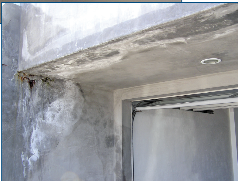
Figure 13 - Exterior leaking, efflorescence, structural cracks, and rust.
