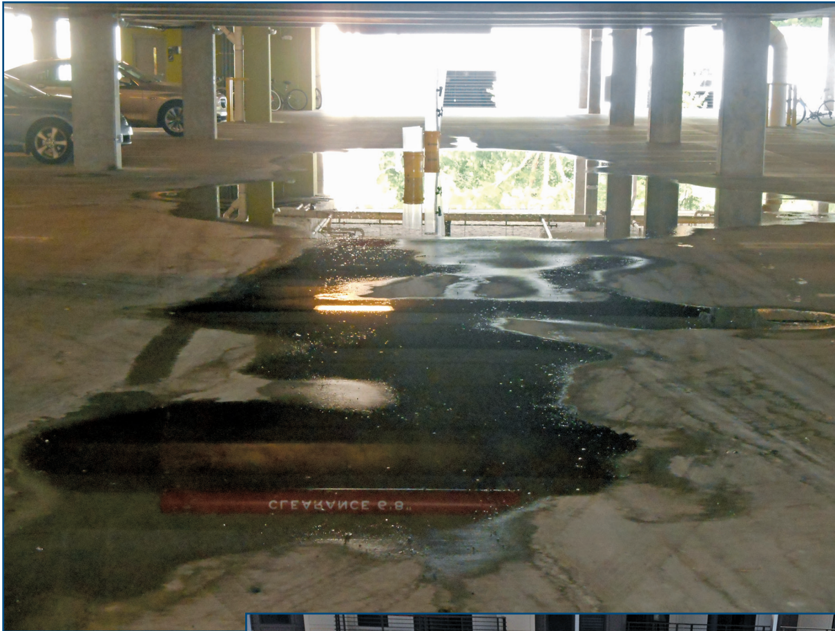
Figure 14 – Water intrusion into parking structure.
