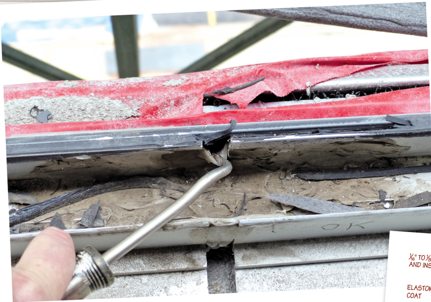
Figure 5 – Failure of retrofitted sealant at splices.
