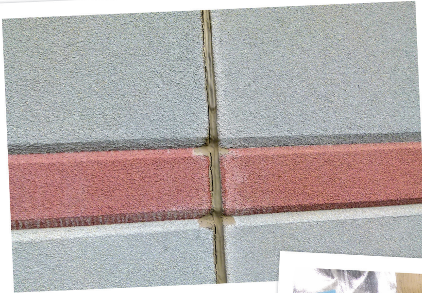
Figure 2 – Failed sealant between EIFS panels.
