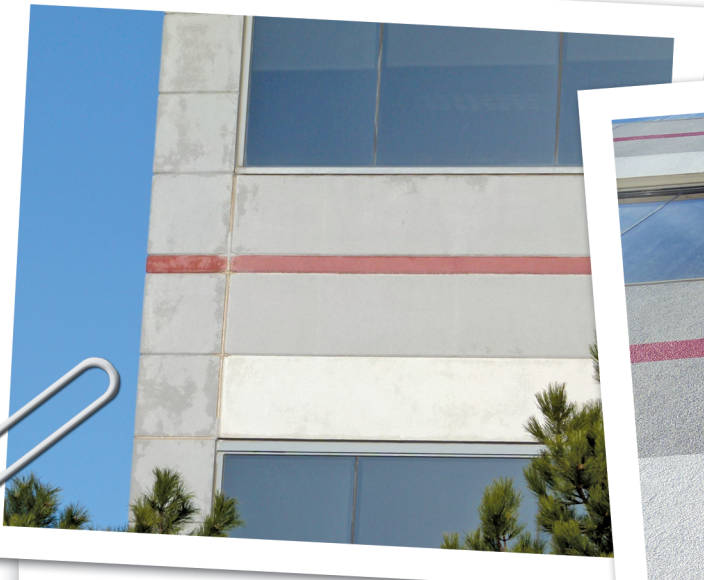
Figure 7 – Original EIFS cladding.
