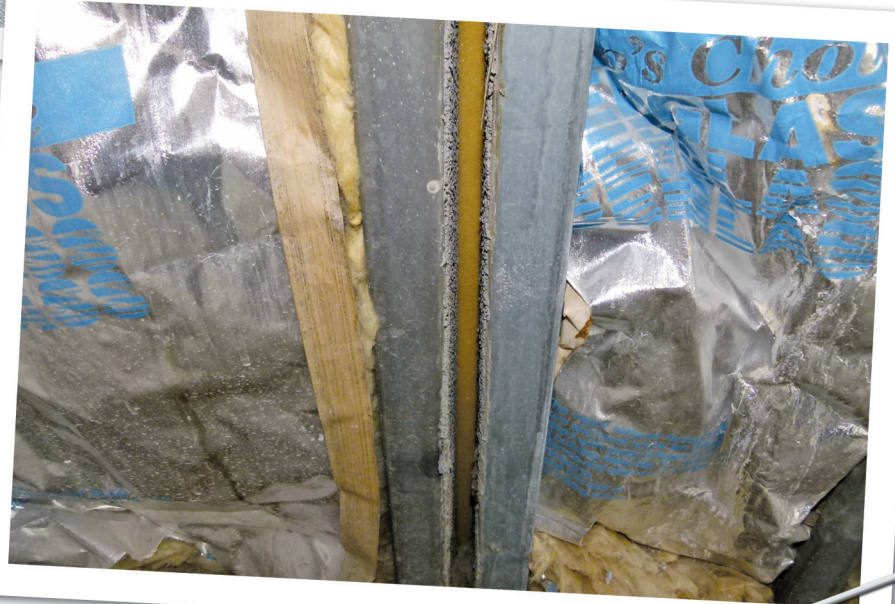
Figure 3 – EIFS base and finish coats extended onto studs.
