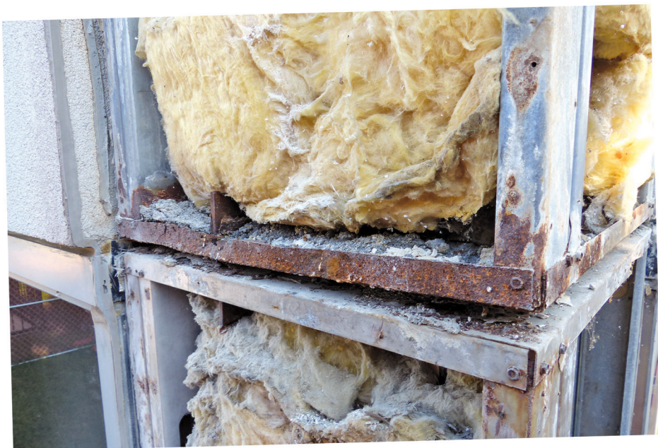
Figure 21 – Corroded light-gauge steel-framing members.
