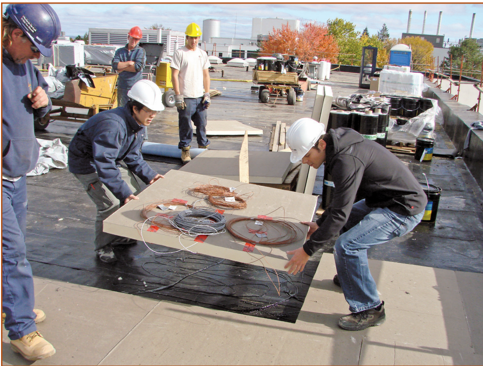
Figure 7 – Installation of heat flux meters and thermocouple instrumentation to monitor VIP composite and polyiso performance.
