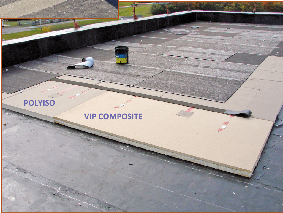
Figure 4 – Installation of polyiso and VIP composite side by side as a point of comparison.
