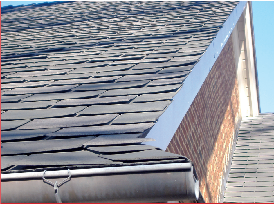
Figure 4 – Warped polymer shingles detract from a roof’s appearance and impact its watertightness. Photo courtesy of Alan Buohl, GSM Roofing, Ephrata, PA.
