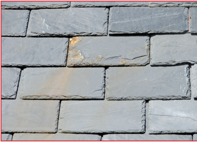
Figure 4 – Rainwater has washed particles of oxidizing iron pyrite down the roof, leaving a very visible rust stain trail.
