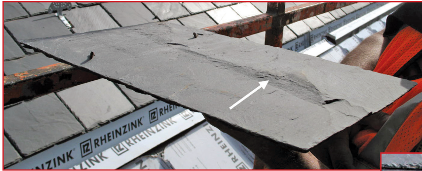
Figure 1 – A cramp on the underside of this slate shingle caused it to stick up and rock from side to side when installed on the roof.
