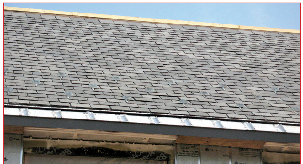
Figure 3 – Numerous slates with raised butt ends detract, aesthetically, from a building's appearance and may impact the longevity and watertightness of the roof system.
