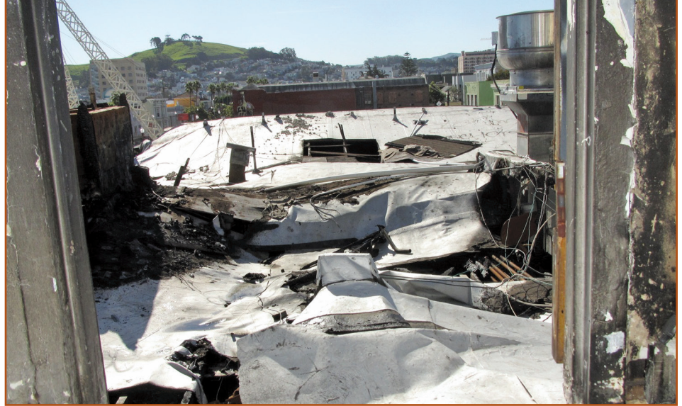
Photo 3 – The roofing system was destroyed by the fire and by the high volume of water deployed by the firefighters.
