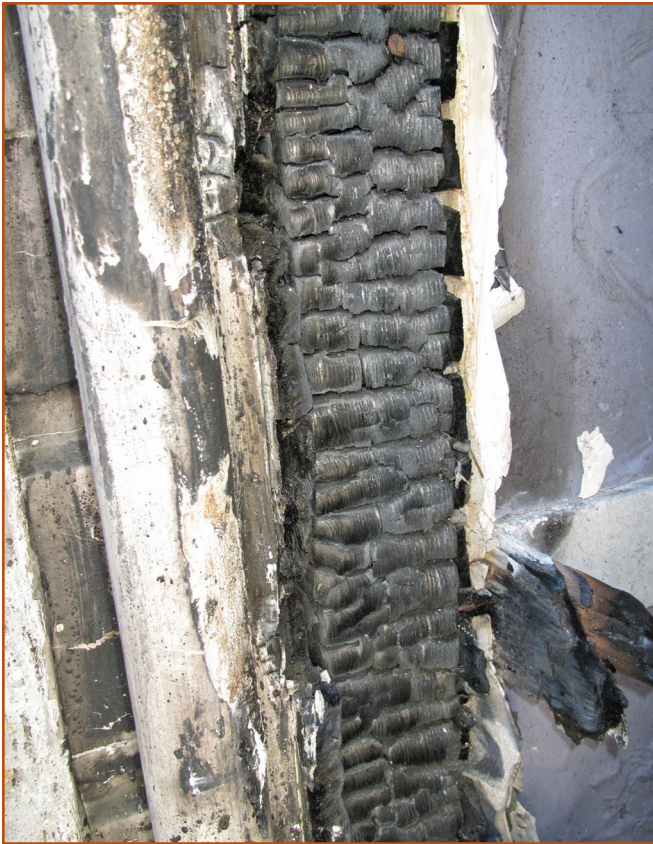
Photo 9 – Lath and plaster walls at occupied third-floor apartments burned from the inside out. (Note the burnt ends of the wooden lath at the right side of this fire-damaged wood stud.)
