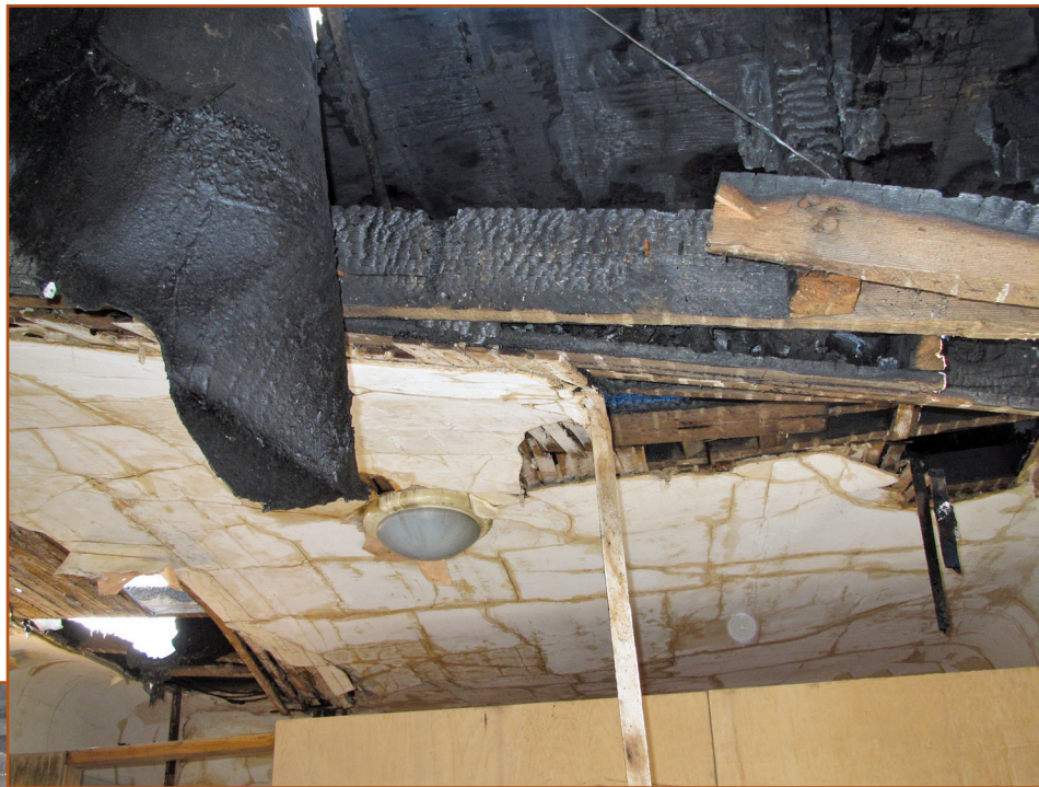
Photo 5 – The stealthy “top-down” fire dropped burning materials and smoke into occupied apartments below. (This lath and plaster ceiling exhibits stress cracking from the many thousands of gallons of water used to fight the fire.)
