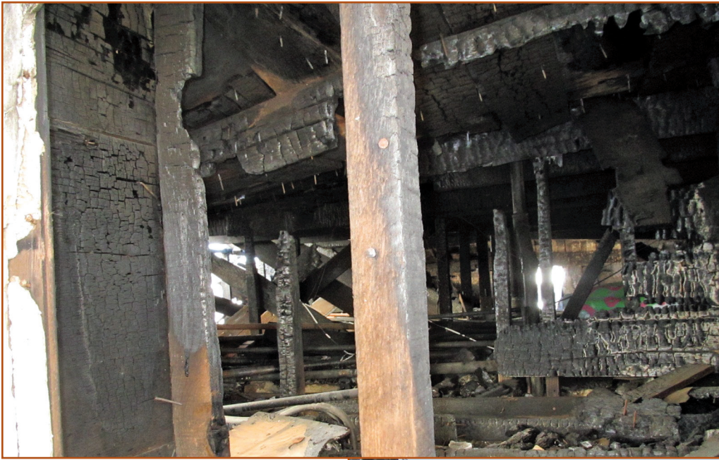
Photo 2 – The fire extended “to and throughout the common attic space above.”
