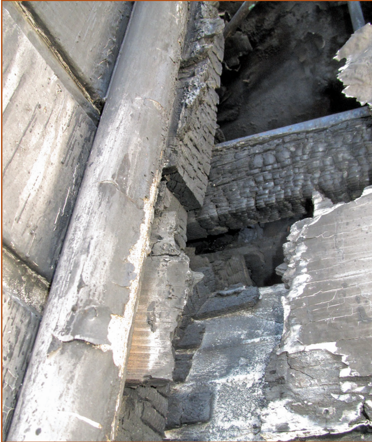
Photo 8 – The attic fire readily dropped into the third-floor wall assemblies (lath and plaster) due to the lack of “bridging” – burning the walls from the inside out, per Photo 9.
