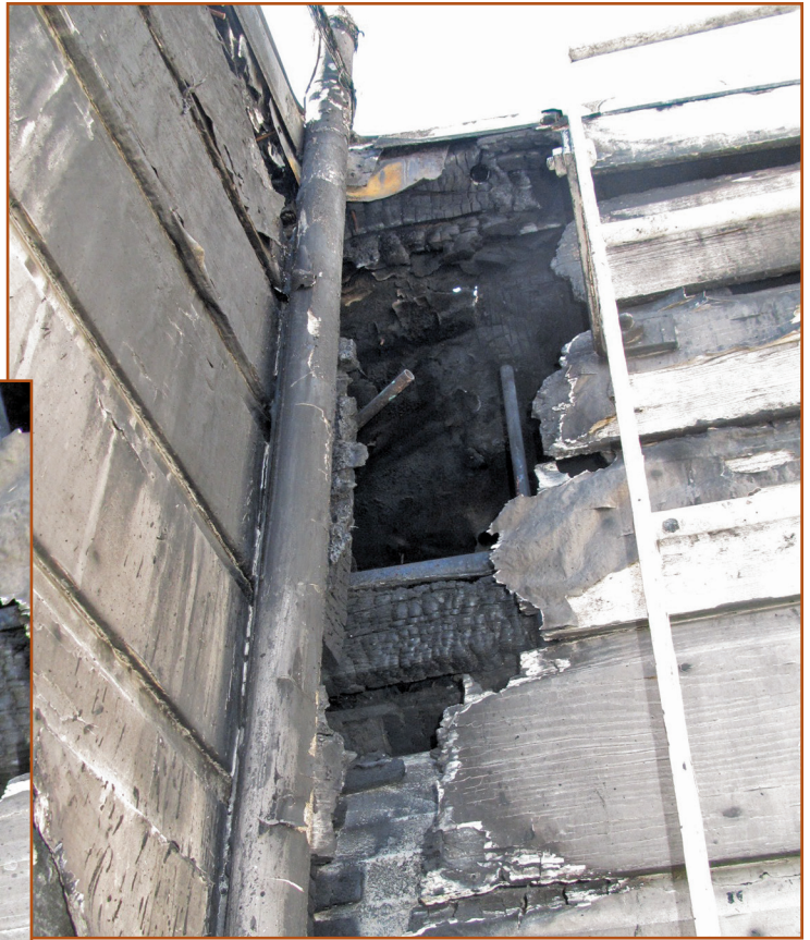
Photo 7 – The attic fire readily dropped down into this third-floor wall due to the lack of “bridging” called out in the 1906 Building Law of the City and County of San Francisco.
