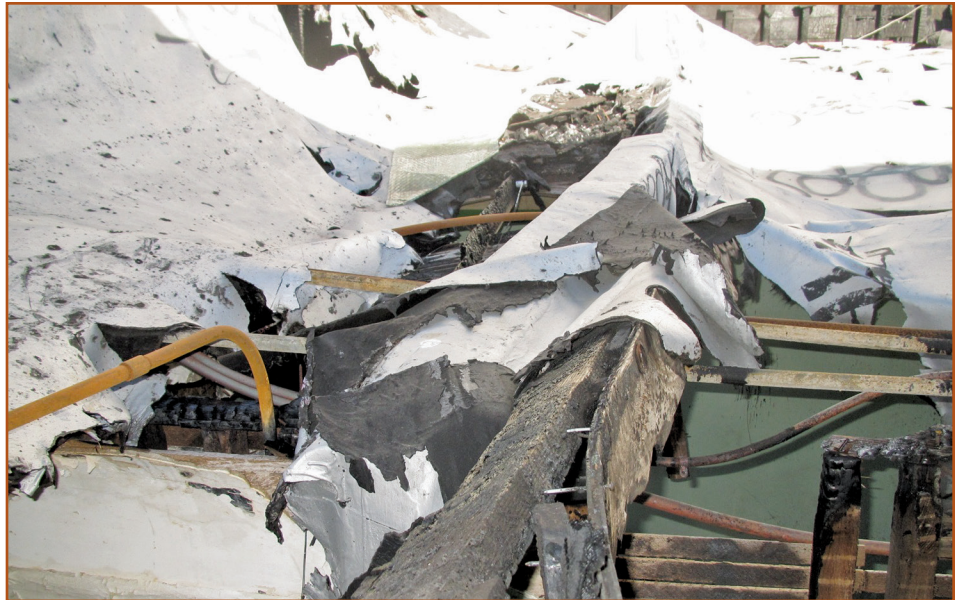
Photo 4 – The “top-down” attic fire dropped burning materials and smoke into occupied apartments below.
