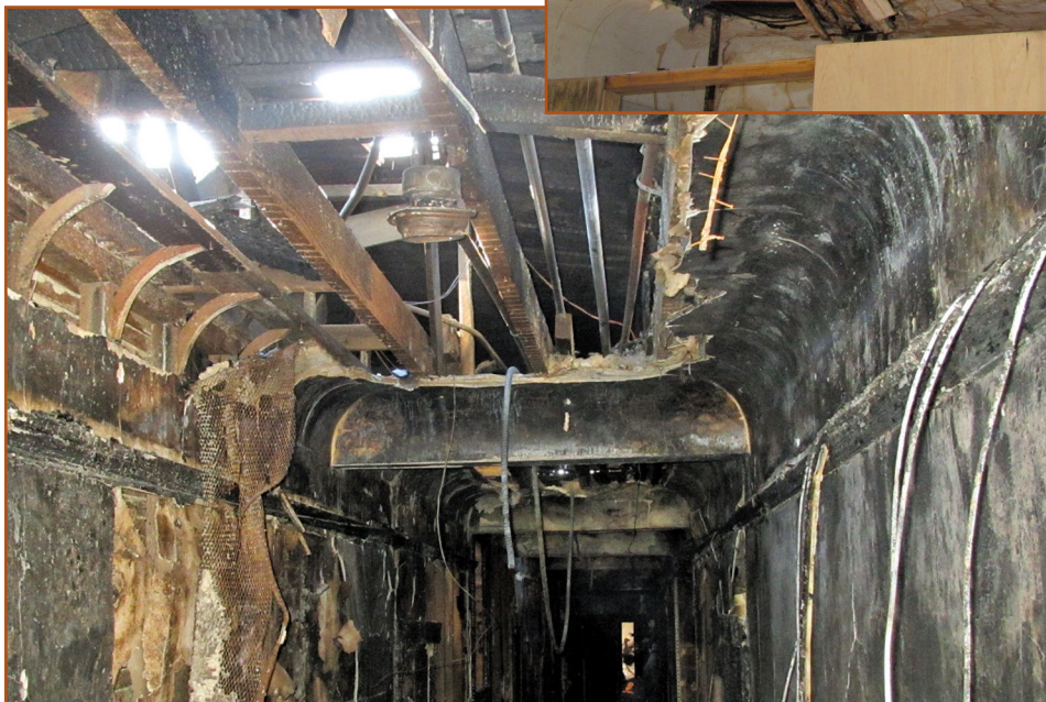
Photo 6 – The attic fire filled the third-floor hallways with smoke, closing off escape routes for the trapped tenants.
