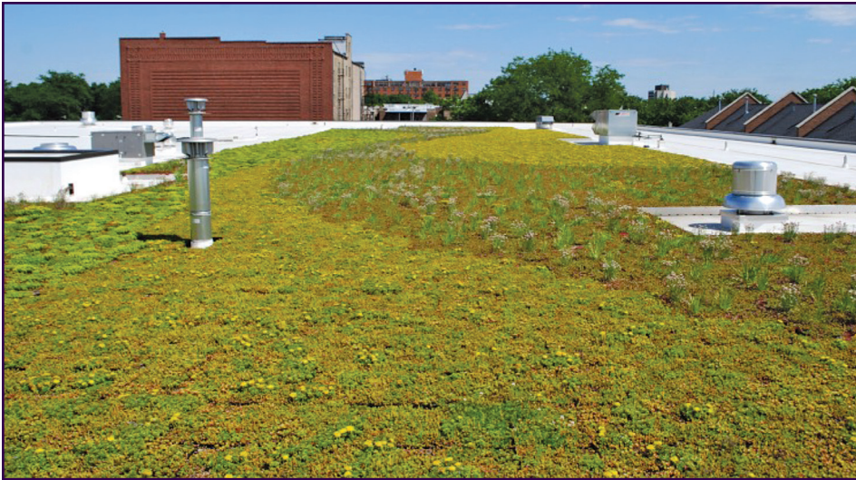
Figure 9 – Vegetative roof system.
