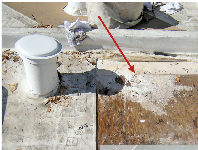
Figure 3A – A “soft spot” (red arrow) found next to an improperly terminated gas vent.
