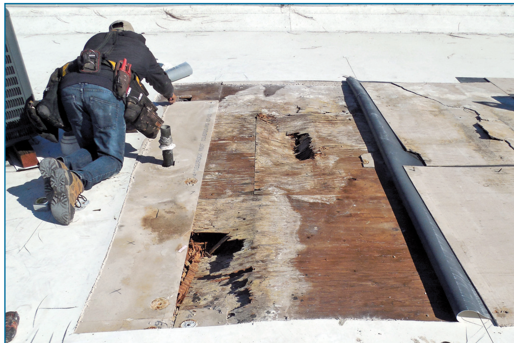
Figure 8 – An area of concentrated decay.
