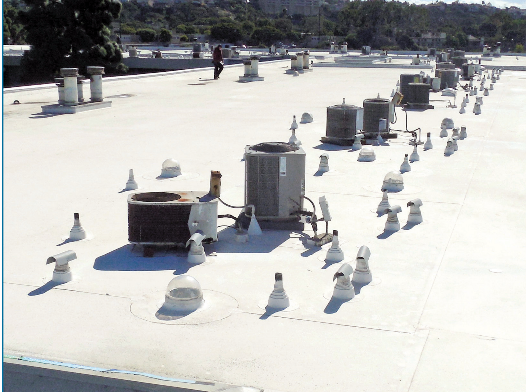
Figure 2 – A high concentration of exhaust vents on the roof of a three-story apartment building.
