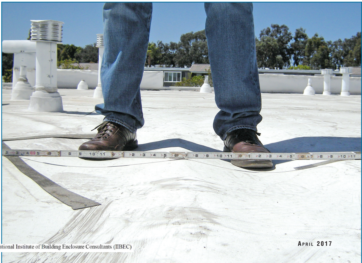
Figure 1 – Serious condensation problems usually start with someone noticing a soft spot.
