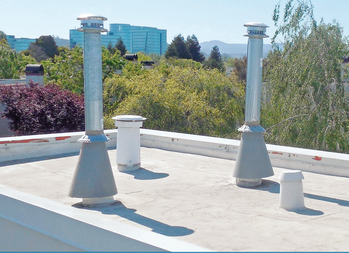
Figure 7 – Two properly extended and terminated gas vents.
