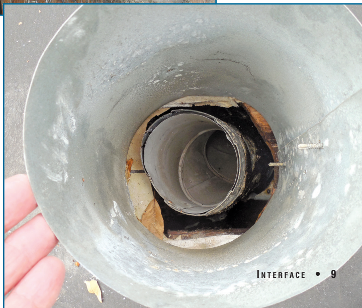
Figure 3B – A gas vent improperly terminated inside the roof flashing assembly very near deck level.
